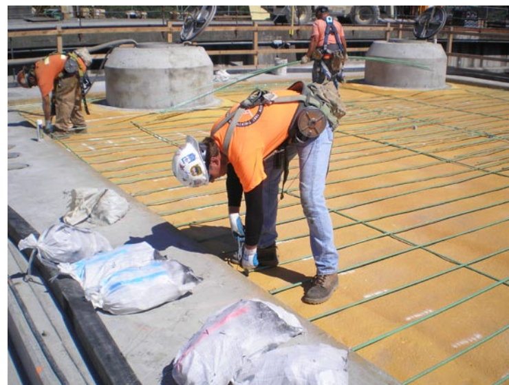
Workers place approved rebar into the bottom of a Hood Canal Bridge pontoon, July 6, 2007.
