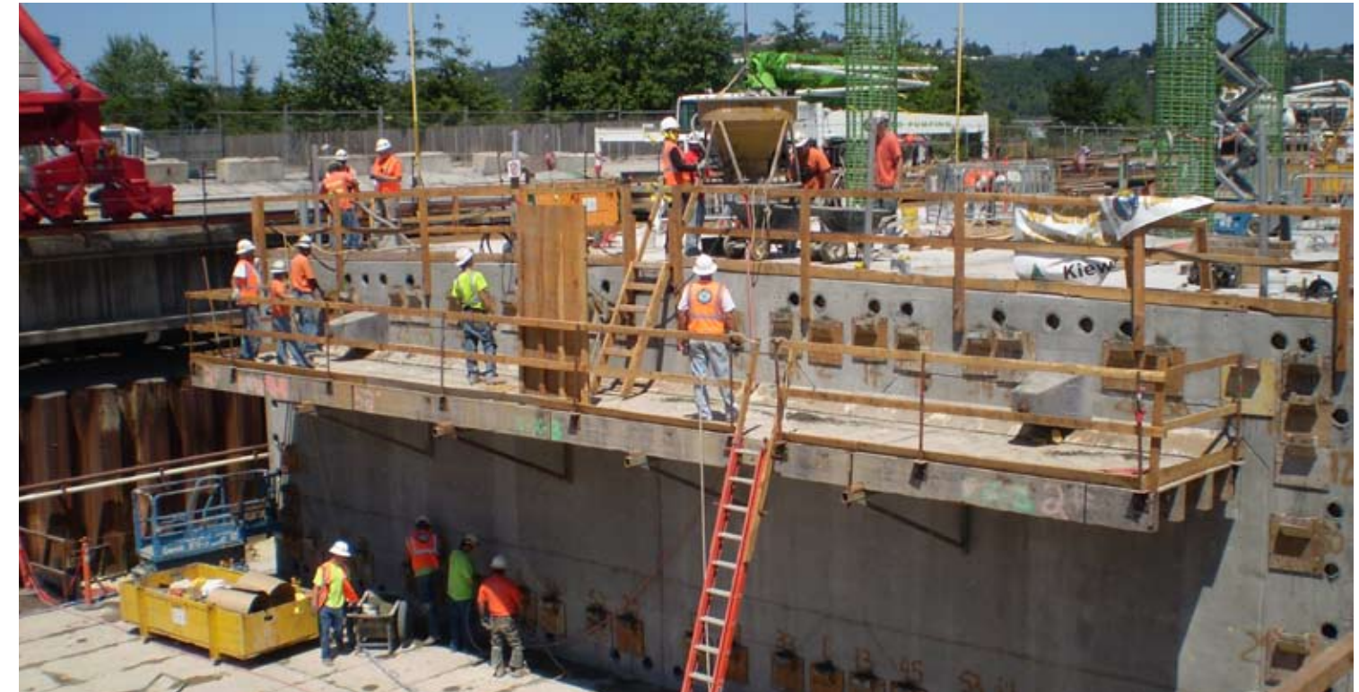
K-G crews place concrete on the west end of pontoon U to protect the ends of the longitudinal post-tensioning strands. July 10, 2008
