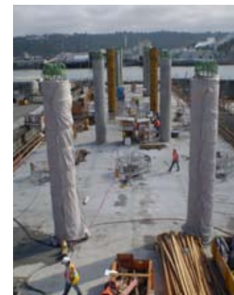
With just days to go before the fourth cycle float-out, pontoon U is prepped for its trip to Seattle. July 21, 2008.
