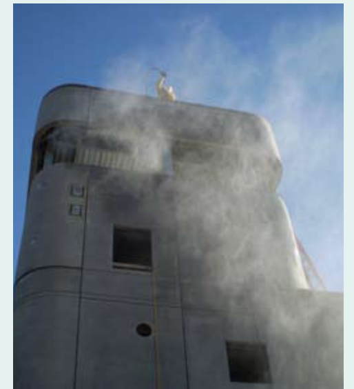
Crews pressure wash the east control tower in preparation for painting. July 11, 2008.
