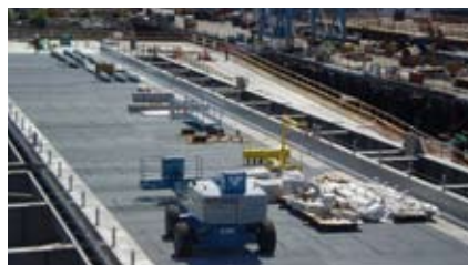
Materials for the east control tower catwalk and lift spans are staged on the recently installed lift spans. July 9, 2008.
