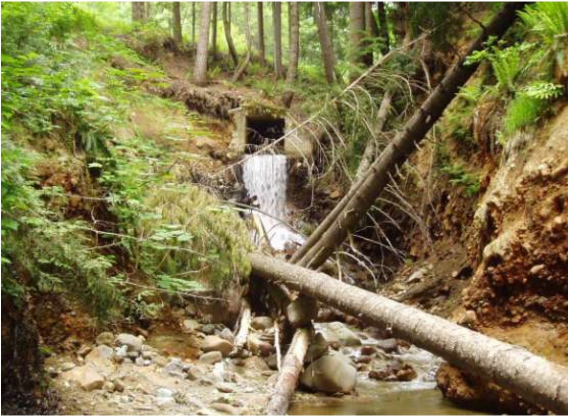
Figure 2. Channel Incision at the Culvert Outlet.
