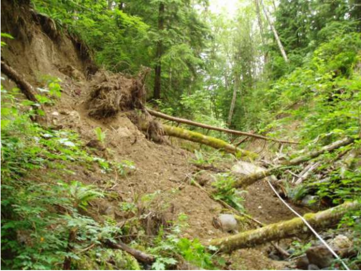
Figure 9. Failing Banks in the Gully Downstream of SR 410.
