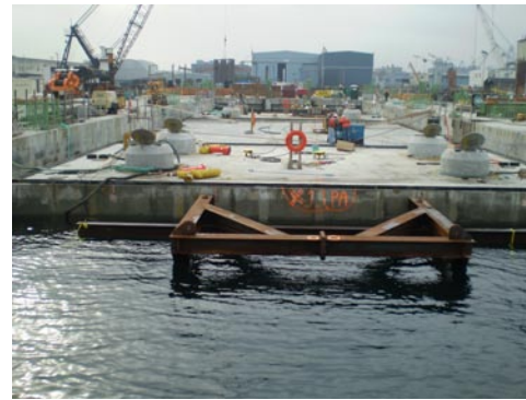
Crews prepared pontoon YF for joining, including ballasting the pontoon with water, October 31, 2007.
