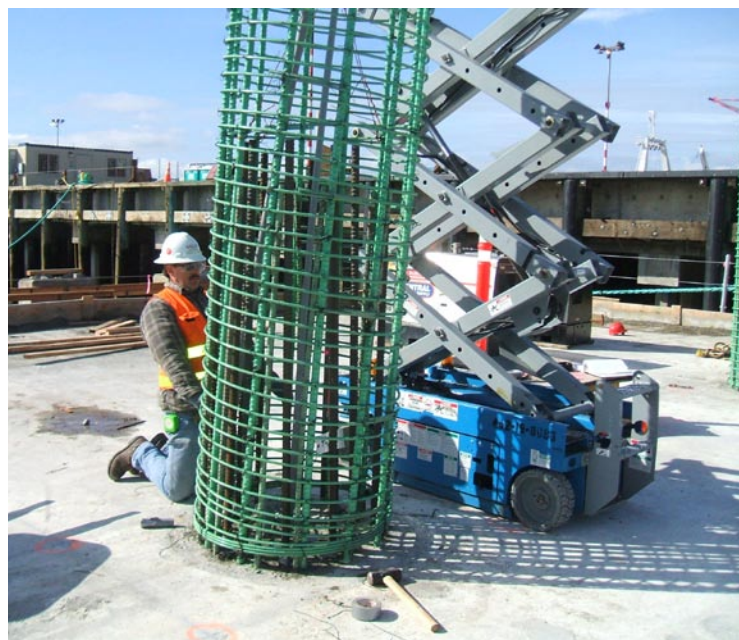
Crews install conduit for road deck lighting through the pontoon T column, March 21, 2007.
