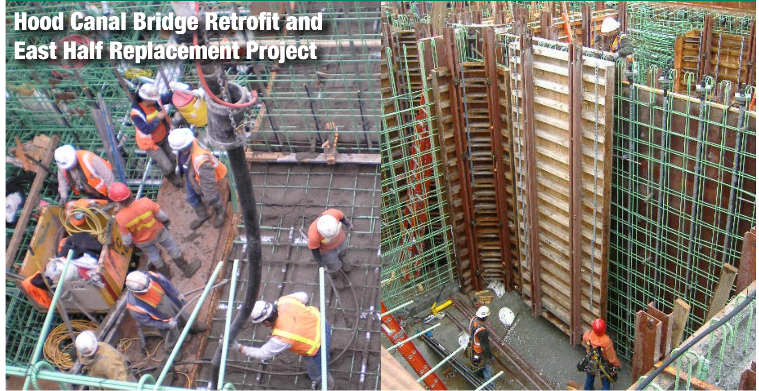
(Left) Crews place concrete for base slab pour on pontoon NA, March 9, 2007. (Right) Crews set the wall panel on pontoon NB, March 19, 2007.
