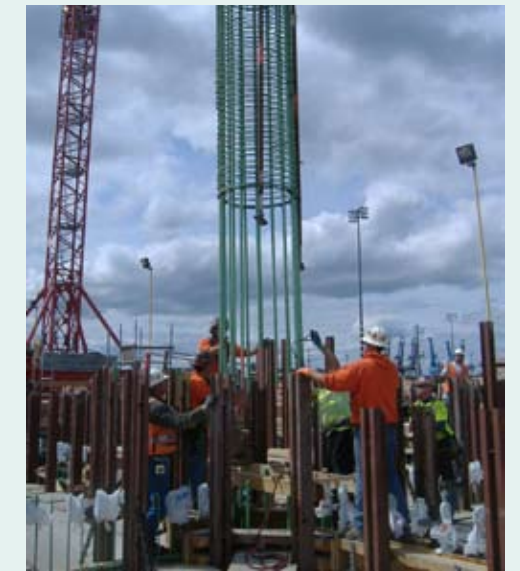
A reinforced rebar cage is placed on pontoon U at CTC. May 1, 2008.
