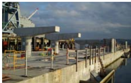
K-G crews will begin roadway installation on the PB pontoon, following the construction of supports and columns. May 1, 2008.
