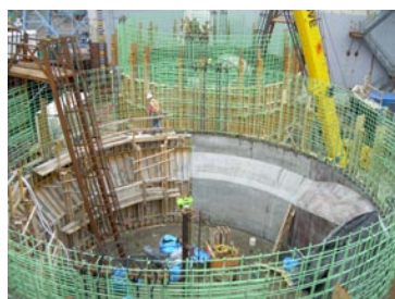
Workers strip inside forms of lower wall on a 60-foot anchor. Jan. 22, 2007.
