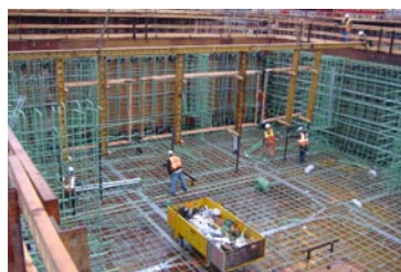
Workers place studs for wall rebar templates on pontoon YD. Templates help support the rebar and will be removed after the base slab pours are complete. Jan. 18, 2007.
