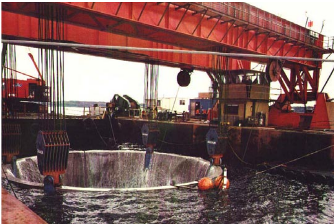
Cable blocks lower an anchor after the ballast (crushed rock materials used to stabilize the anchor) is placed inside. Approx. 1980
