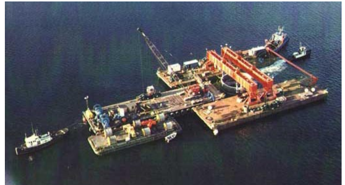
Tug boats tow anchors to the bridge to be set on the Canal floor. Approx. 1980
