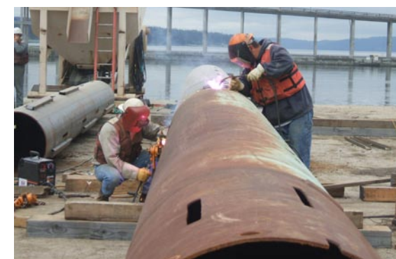
Workers fabricate the tremie pipe for anchor ballasting. Rock is placed through the tremie pipe and down to the anchors on the Hood Canal floor. June 14, 2007.
