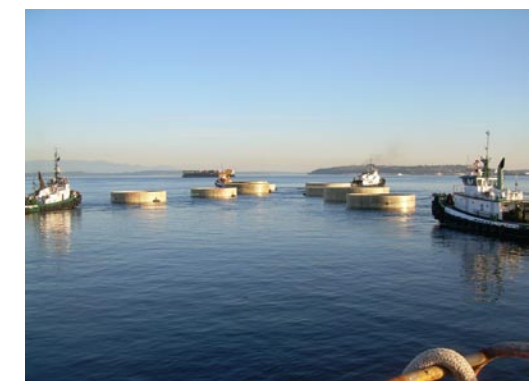
(Top) Water floods the dry dock. June 20, 2007. (Bottom) Tug boats separate the anchors before their journey to Port Gamble. June 20, 2007
