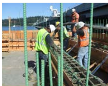
Workers place concrete in the lower wall forms of the west-half electrical building, August 14, 2007.
