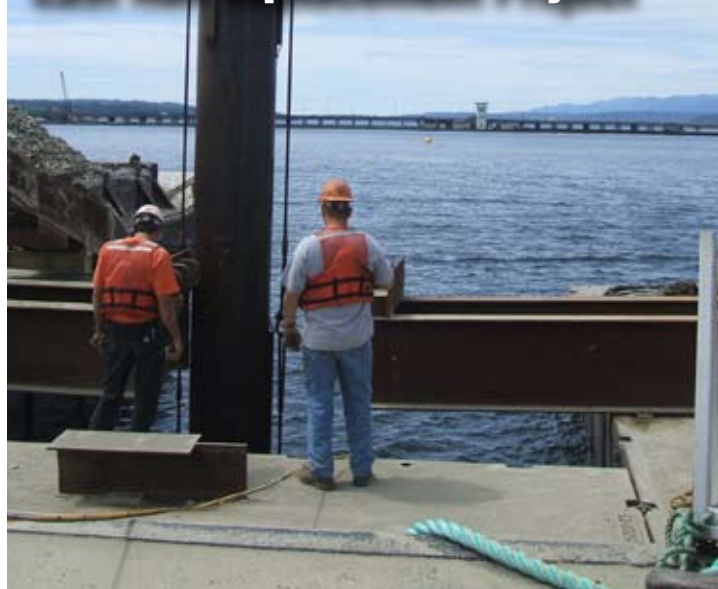
Crushed rock flows down through a large pipe to the anchor at the bottom of Hood Canal, August 2007.
