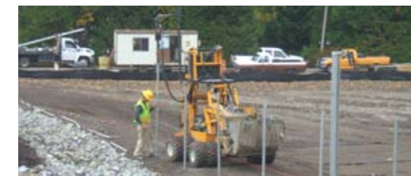
Worker installs fencing around Park-and-Ride lot and around the slope area, October 25, 2006.
