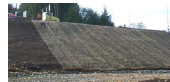
Workers install erosion mats along the north side of the east approach to the bridge, October 23, 2006.
