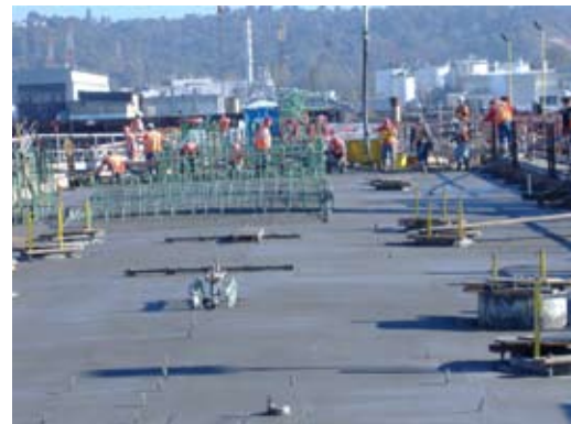
(Far left) Workers pour concrete around post-tensioning tendons on pontoon PA, October 19, 2006. (Left) Workers pour concrete for the last section of the top deck on pontoon PB, October 11, 2006.
