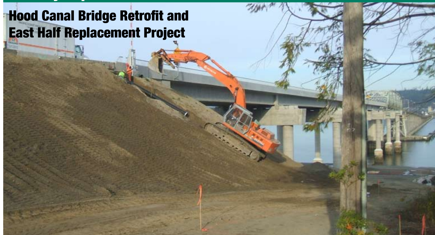
Crews install drain pipe as part of storm water runoff system for SR 104, October 3, 2006.
