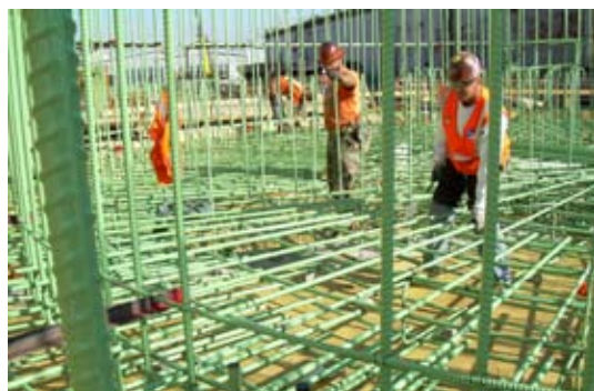
Ironworkers install next layer of rebar for anchor floor and walls, October 13, 2006.
