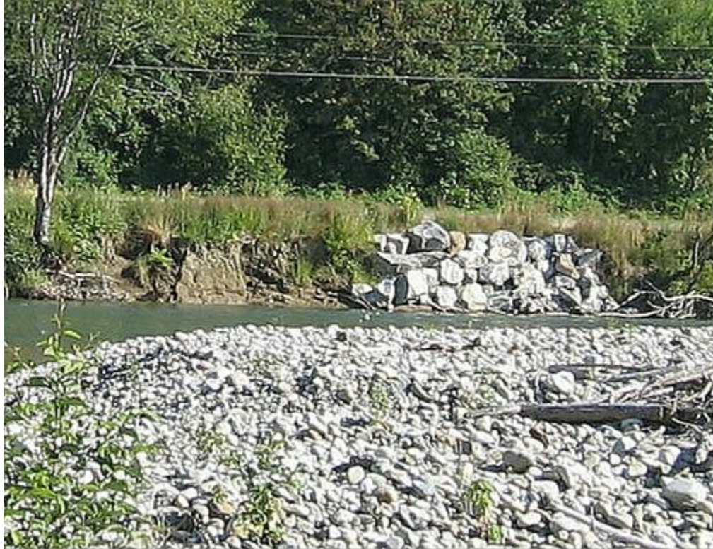
Figure 5. Bank erosion downstream of 2004 repair.
