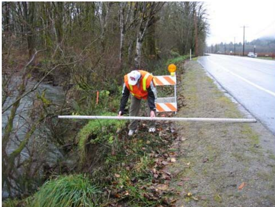
Figure 4. Bank erosion progressing to within eight feet of the roadway (11/23/04).
