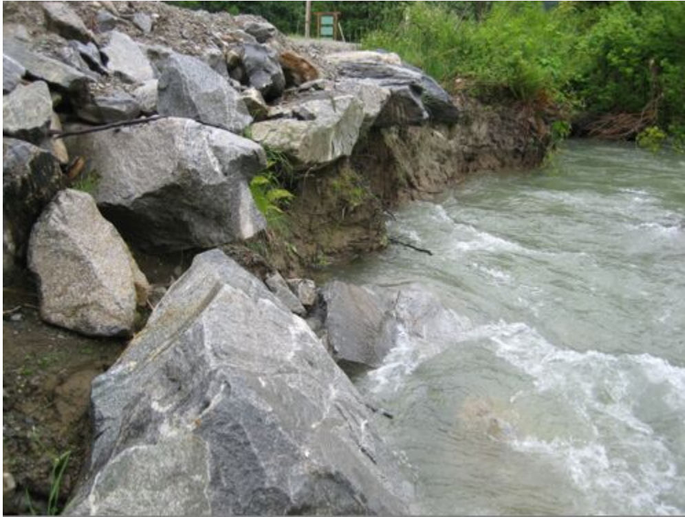
Figure 7. Undermining of 2006 repair.
