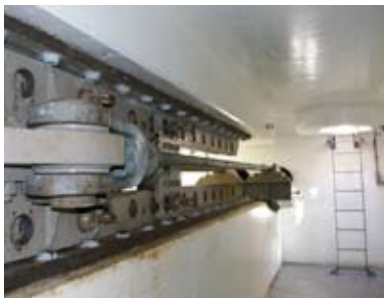
A close-up look at a new anchor cable connection on the east half. Aug. 20, 2009.
