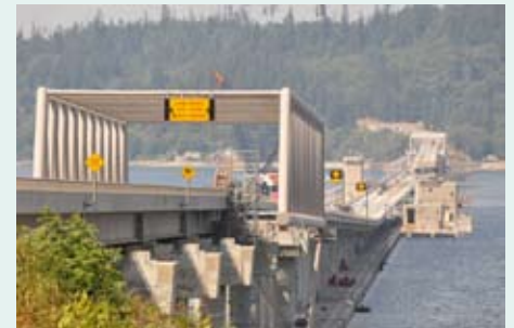
The new east half of the bridge features wider, safer lanes and a new truss. Aug. 5, 2009.
