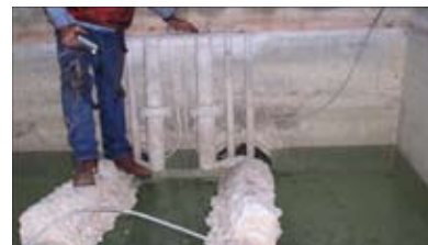
Oxidizing zinc anodes near the rectifier produce a white crystalline substance.
