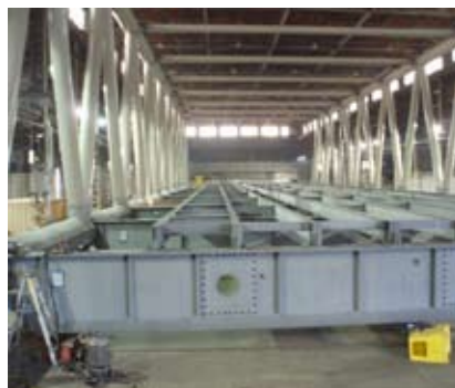
Work continues on the west truss of the Hood Canal Bridge. The truss is expected to be completed in April 2008. The 270-foot-long truss will connect the bridge's floating pontoons to an approach span in Jefferson County. Feb. 21, 2008.
