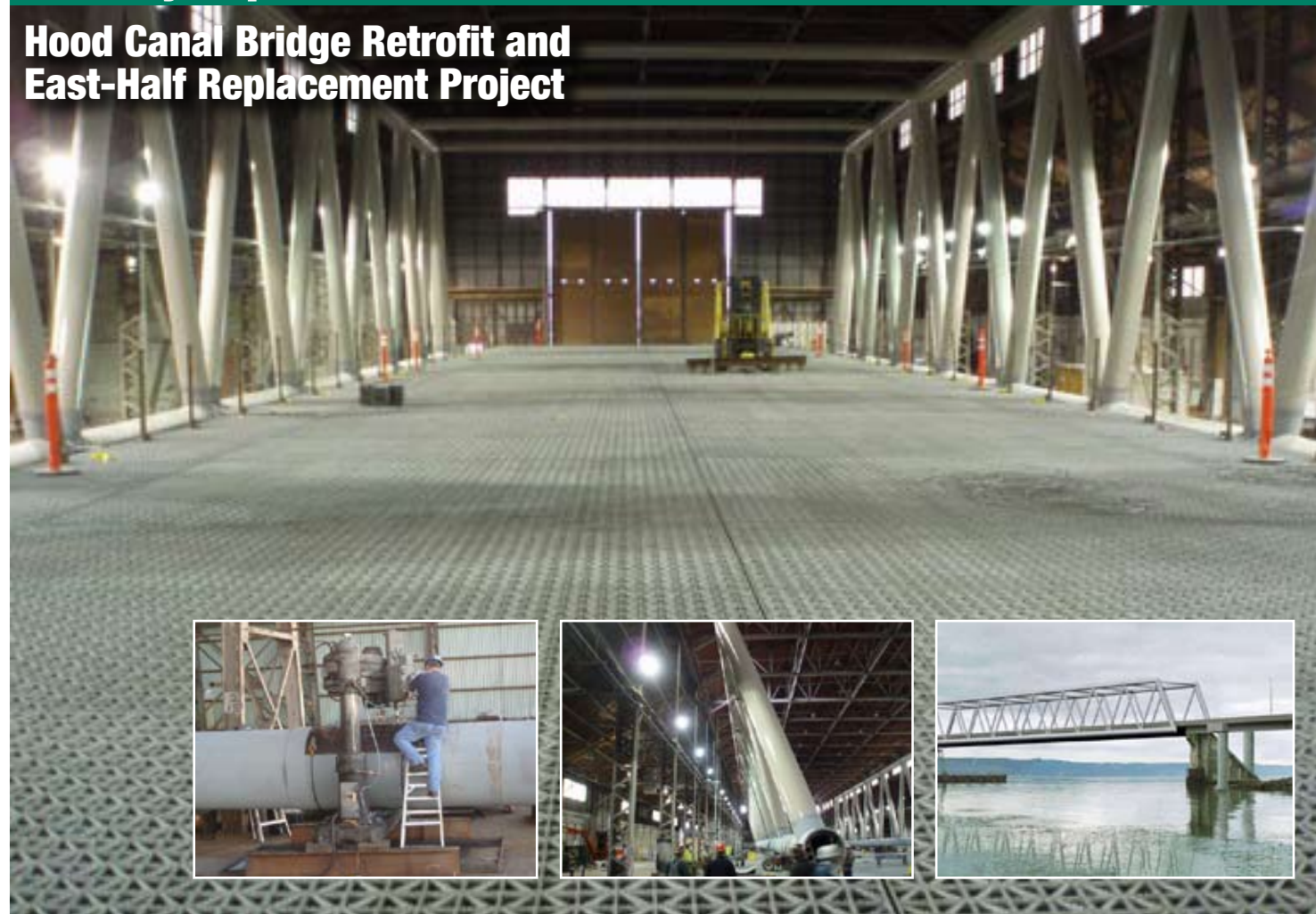
Large photo: The west truss assembly construction is making progress toward completion, the grating that will be its roadway was recently installed. March 19, 2008. Inset photos: (Left) An Oregon Iron Works (OIW) crewmember machines a section of the trusses' bottom chord. Aug. 27, 2007. (Center) Crews watch as a side of the west truss is raised into place at OIW. Jan. 10, 2008. (Right) Here's what the new west truss will look like when it is put in place during the May-June 2009 closure. Photo illustration created Sept. 16, 2006.
