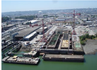
An aerial view of the graving dock at Concrete Technology where 14 new pontoons are being constructed for the east-half of the bridge. July 2006
