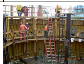
Port of Seattle—Todd Pacific Shipyards: Anchor Construction (21% complete) Workers pour concrete for lower wall section on 46-foot anchor, Nov. 21, 2006
