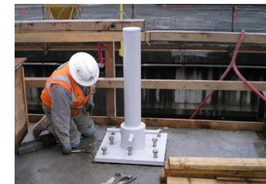
Worker installs a temporary bollard on pontoon PA. Tow ropes attach to the bollards from the tugboats when the pontoons are towed out of the graving dock, Nov. 22, 2006.
