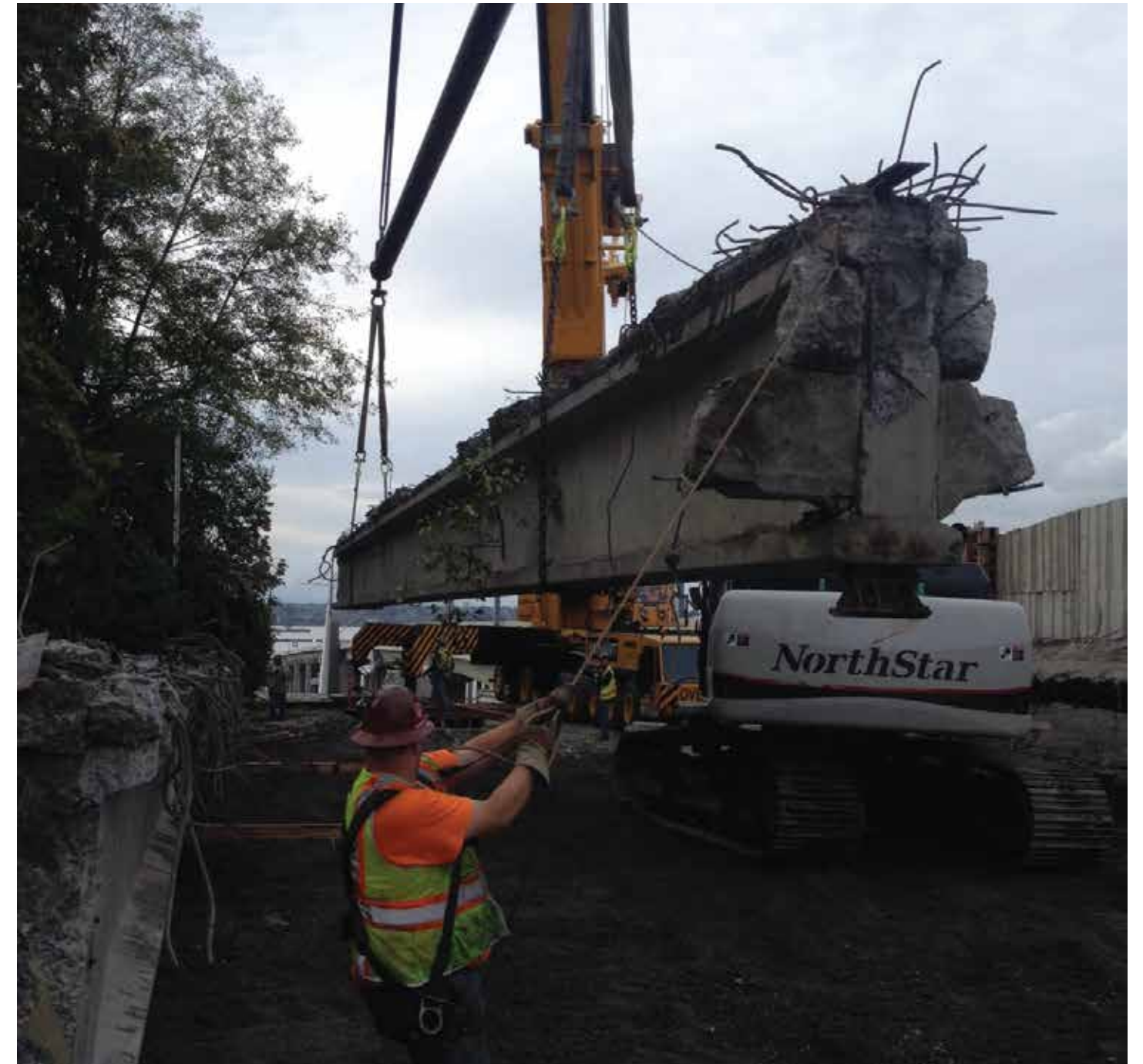
Crews remove girders from the old floating bridge approach in Medina. Photo taken: Oct. 7
