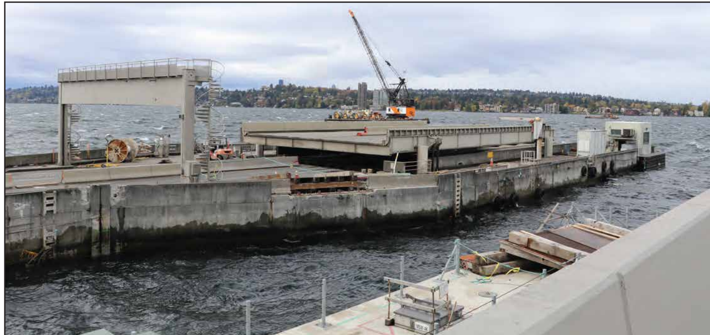
Pontoons that supported the drawspan on the old floating bridge are the last to remain in their original position prior to being towed from Lake Washington. Photo taken: Oct. 8
