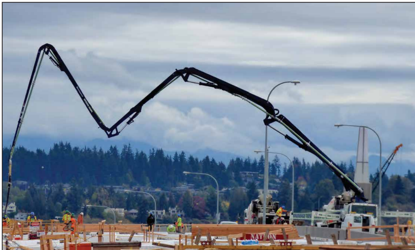
Crews position a concrete boom on the westbound lanes of the new floating bridge in order to pour a section of roadway deck for the new West Approach Bridge North. Photo taken: Oct. 10
