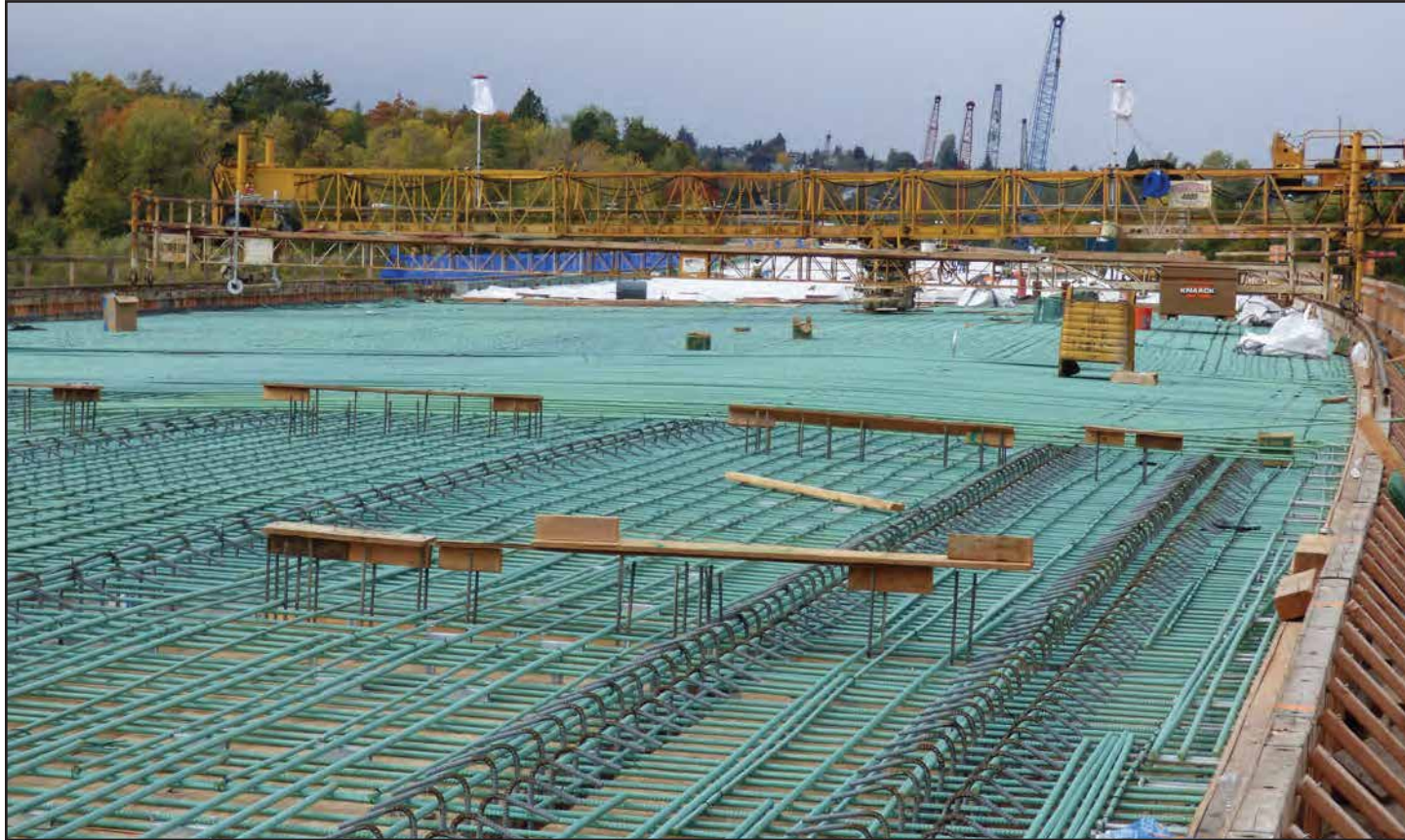
A grid of rebar awaits concrete pours for the West Approach Bridge North roadway deck. Photo taken: Oct. 8
