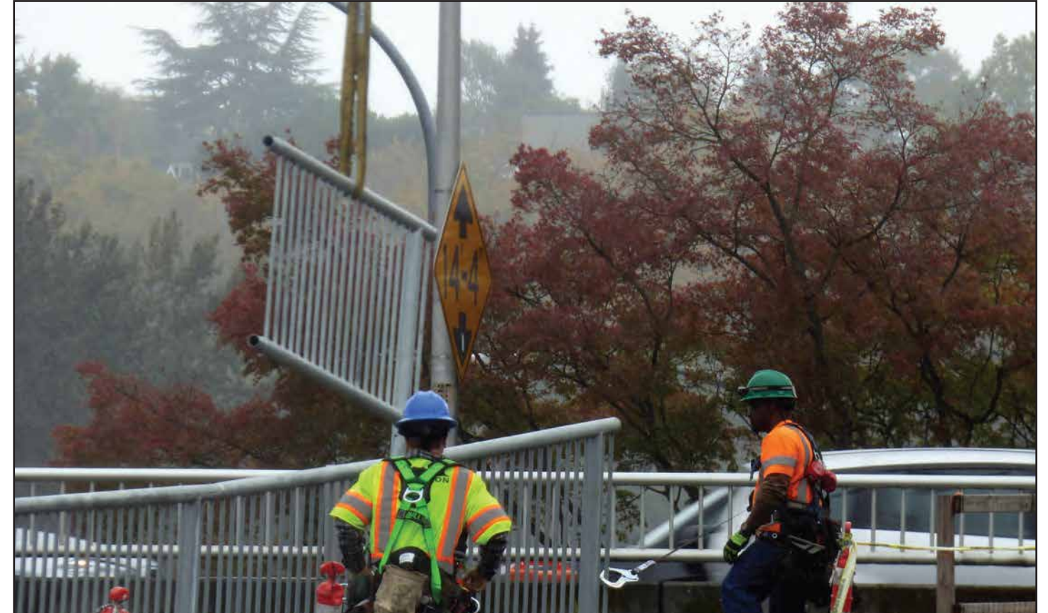
During an Oct. 7 - 10 closure of SR 520, crews begin installing railing at the westbound Montlake Boulevard interchange transit flyer stop. Photo taken: Oct. 10
