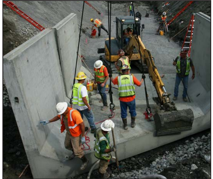
Crews place a section of a fish-friendly culvert near 108th Avenue Northeast during a weekend closure in September.
