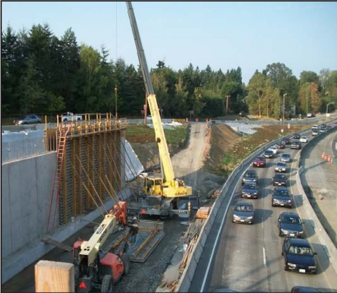
Crews remove a wall form after pouring concrete for a pier wall that supports the new 84th Avenue Northeast lid.
