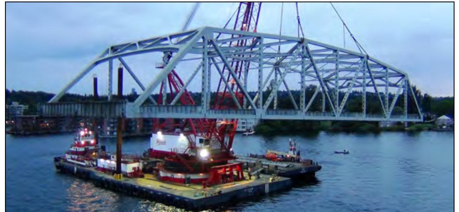
Crews remove the west truss from the old SR 520 floating bridge. Photo taken: May 31
