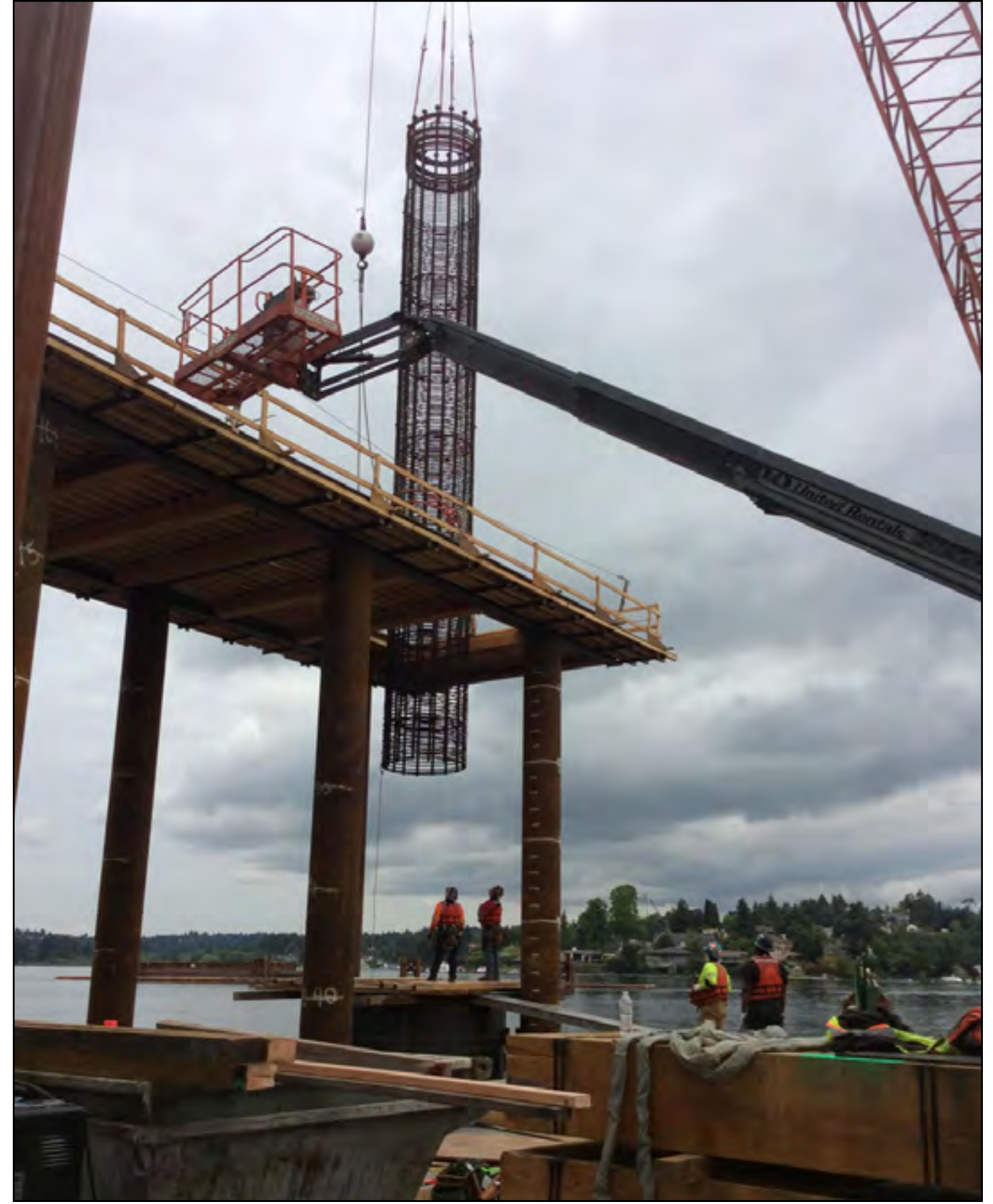
Crews install a rebar cage to strengthen the foundation for the West Approach Bridge North structure. Photo taken: May 24
