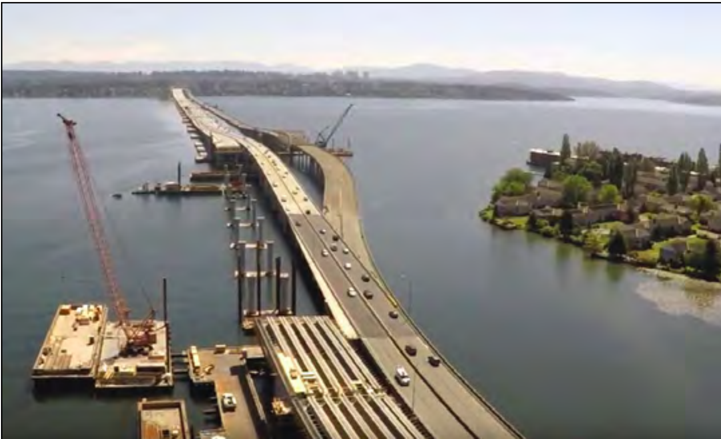
An aerial photo, looking east, with the West Approach Bridge North in the foreground. Traffic flows on the existing west approach bridge between Montlake and the new floating bridge. Photo taken: May 31.
