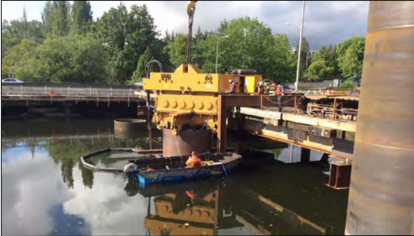
Crews installed the last, few remaining casing for the West Approach Bridge North Project. Photo taken: May 20.
