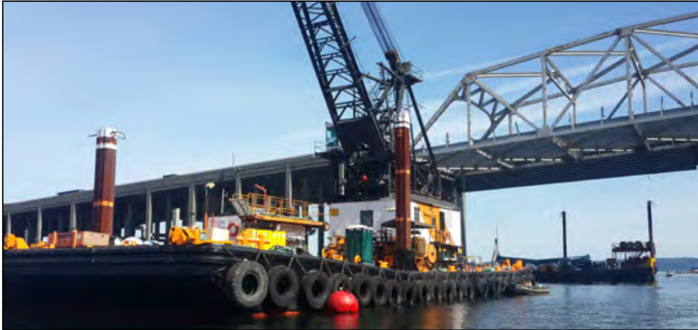
Barge cranes begin decommissioning work on the old SR 520 floating bridge. Photo taken: May 31.
