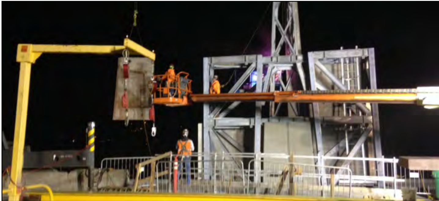
Crews continued to build the Pontoon A north sentinel throughout January. Photo taken: Jan. 18
