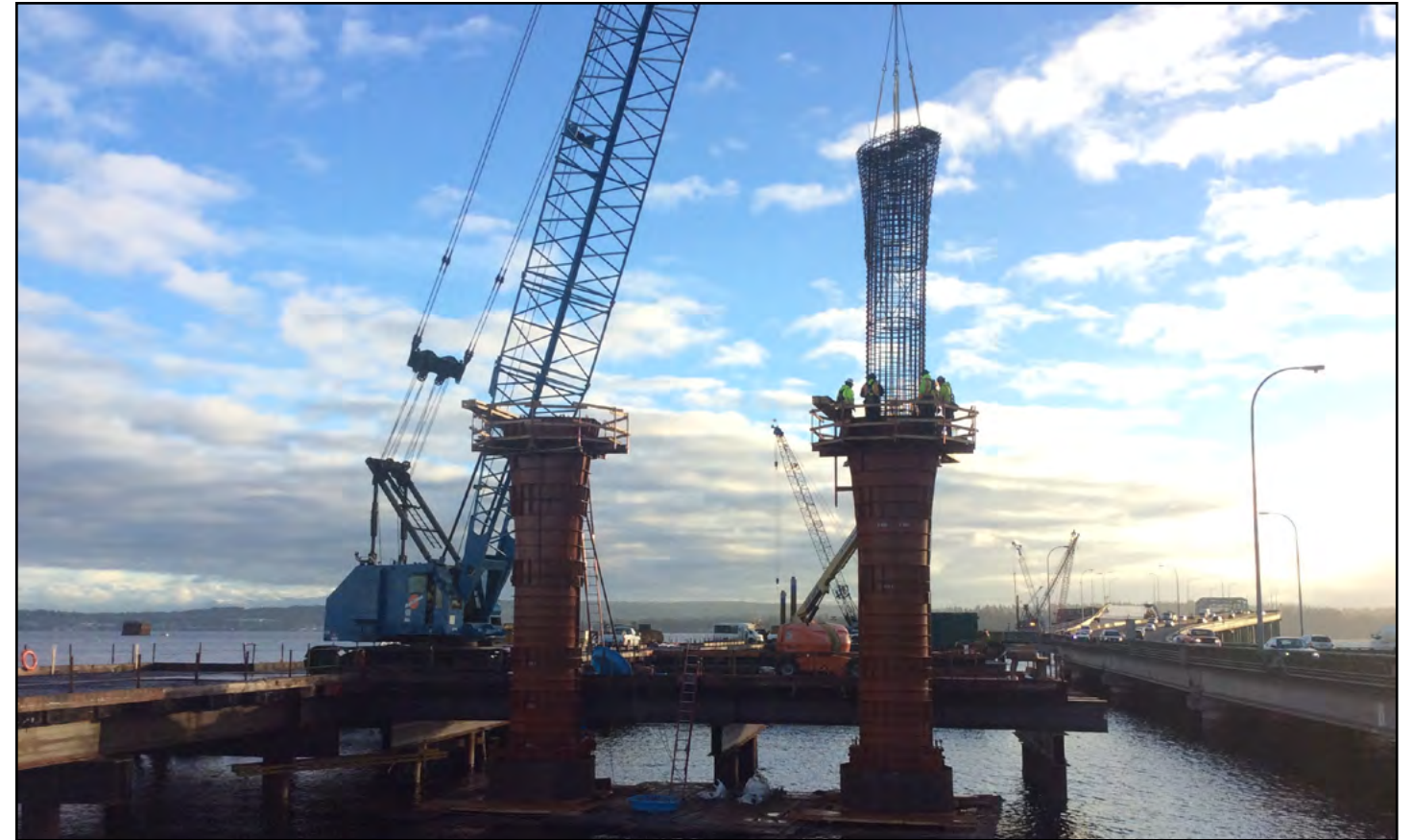
Crews install a column rebar cage prior to pouring concrete into the column forms on the West Approach Bridge North Project. Photo taken: Feb. 23
