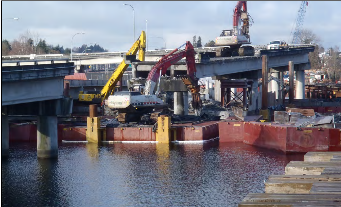
Demolition of the westbound SR 520 off-ramp to Lake Washington Boulevard continues on the West Approach Bridge North Project. Photo taken: Feb. 1
