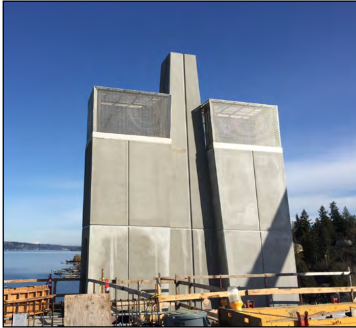
Sentinels mark the beginning and end of the new floating bridge. Photo taken: Feb. 25
