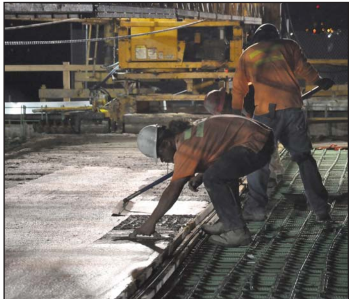
Crews place fresh concrete to form a new lidded overpass on the Eastside.
