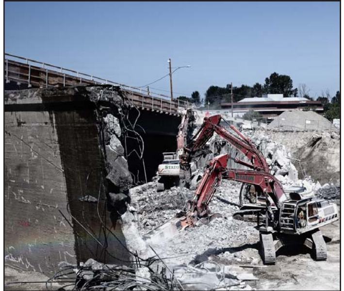
Demolition of the old Bellevue Way overpass takes place during a full weekend closure of SR 520 on Aug. 10-13, 2012.
