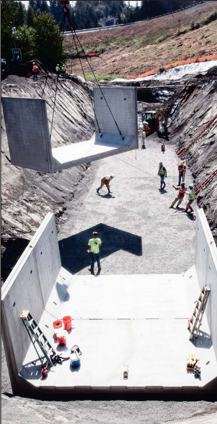
Workers guide a giant concrete culvert section into place. The new culvert will be over 230 feet long and help fish migration.
