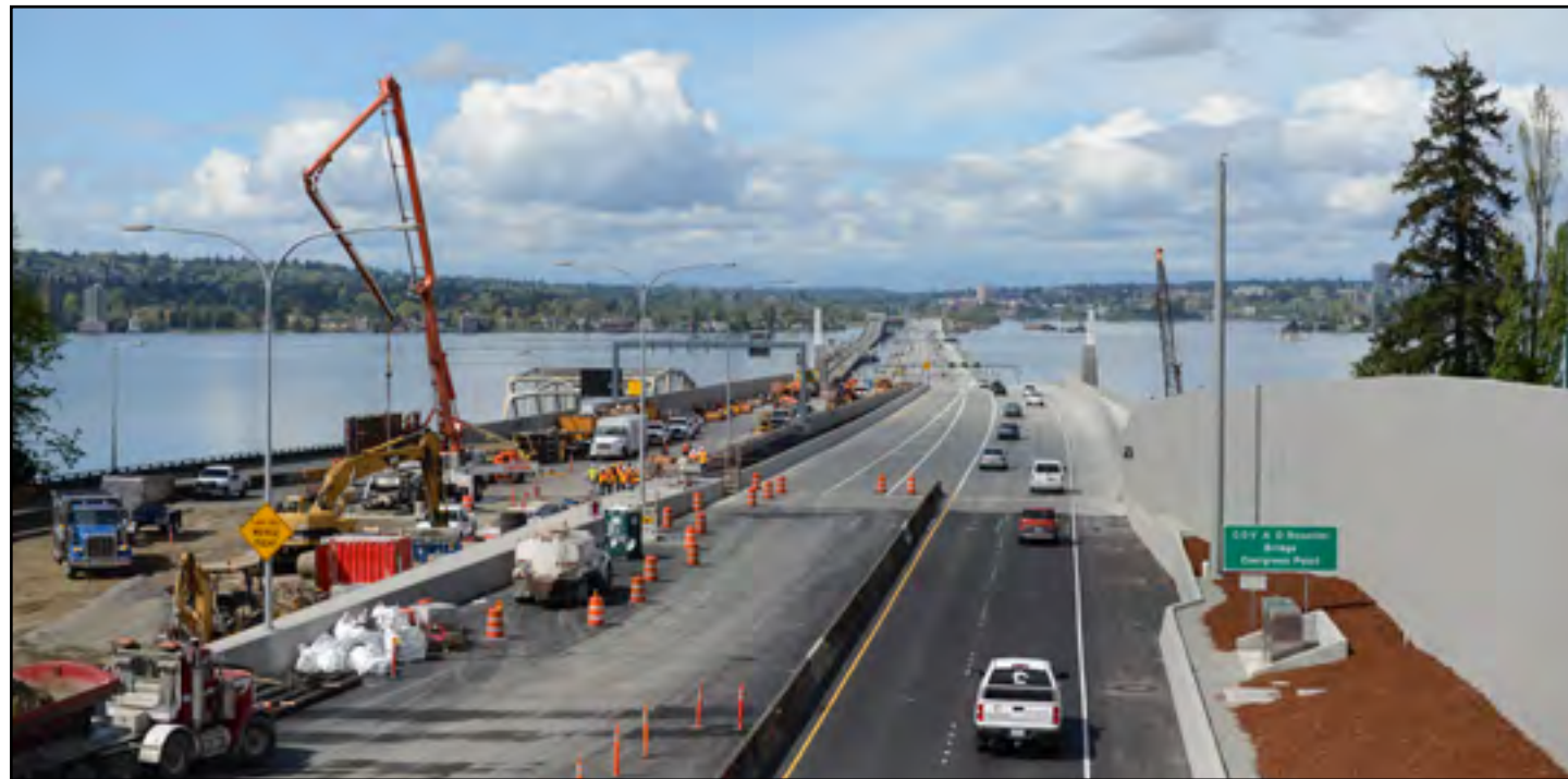
The new SR 520 floating bridge opened to traffic in the westbound direction on April 11, 2016. Photo taken: April 14.
