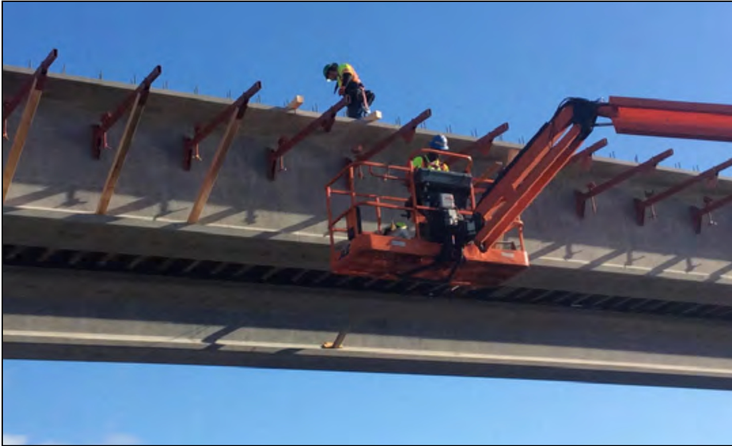
Crews installed brackets to girders to prepare for future roadway deck concrete pours. Photo taken: April 1.
