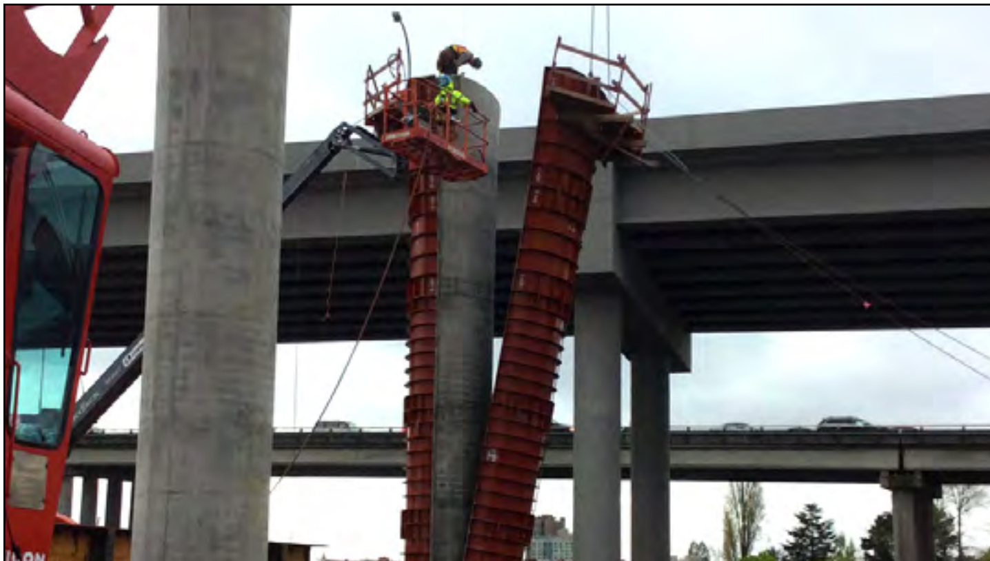
After the concrete has completely cured, crews removed the red column form from columns east of the temporary work bridge. Photo taken: April 1.
