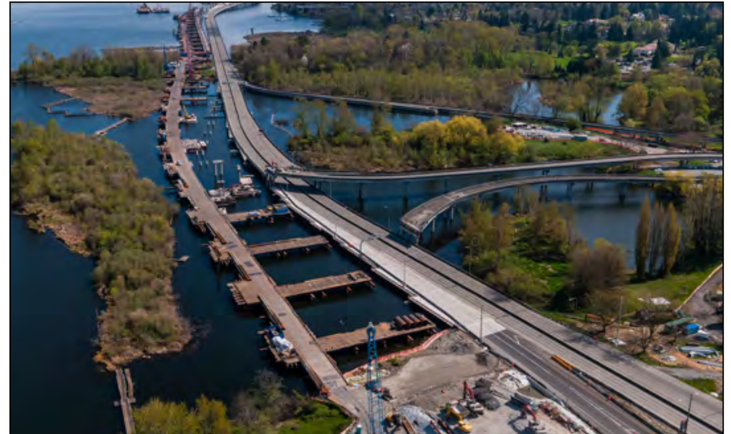
This aerial photo shows progress on the West Approach Bridge North Project. Photo taken: April 2.
