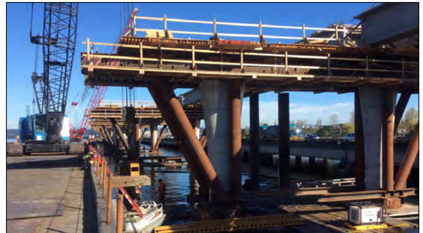
Crews installed falsework on columns east of Foster Island to prepare them for future girder placement. Photo taken: April 1.
