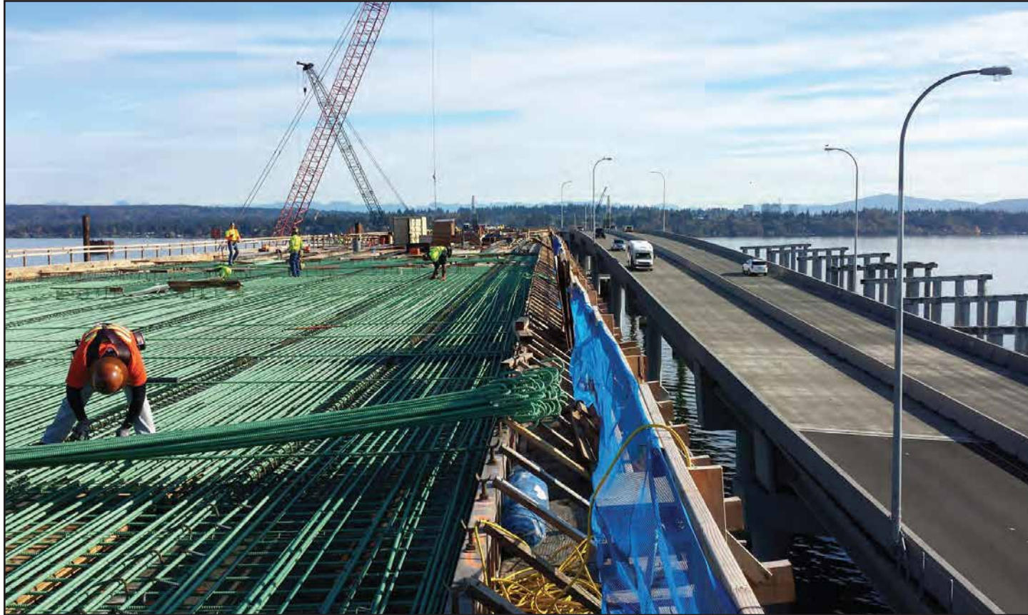
Crews install rebar to reinforce the concrete roadway deck of the West Approach Bridge North. Photo taken: Nov. 4
