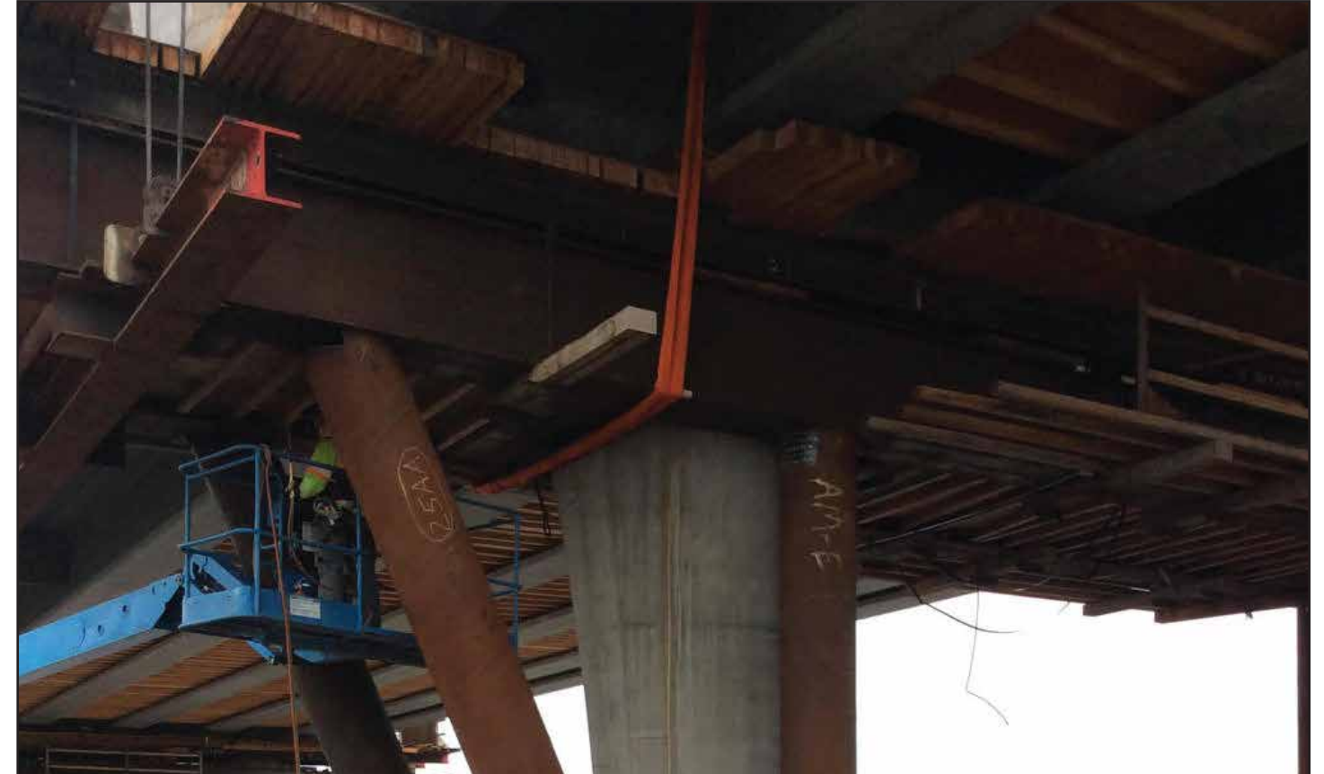
Crews remove falsework from under the West Approach Bridge North. The falsework supports the bridge's girders until roadway deck is poured. Photo taken: Nov. 23
