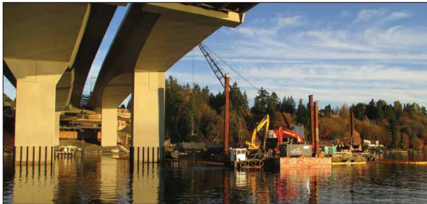
Near Medina, a barge-mounted crane continues underwater removal of concrete columns from the old floating bridge. The new bridge's maintenance facility can be seen, at left, under the east landing. Photo taken: Nov. 3
