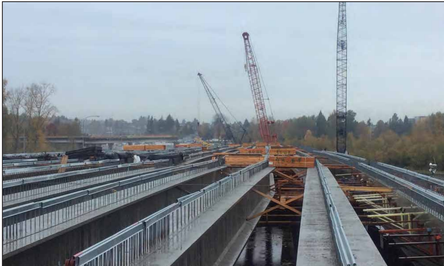
A gray day in Montlake complements these gray, 150-foot-long concrete girders, which form the backbone of the 1.2-mile-long West Approach Bridge North. Photo taken: Nov. 11
