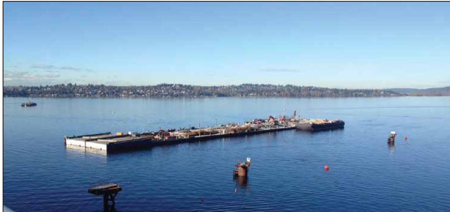
Crews reach the final stage of dismantling the superstructure - the concrete columns and elevated roadway deck - from the old floating bridge's pontoons C, D, X and Y. Photo taken: Nov. 8
