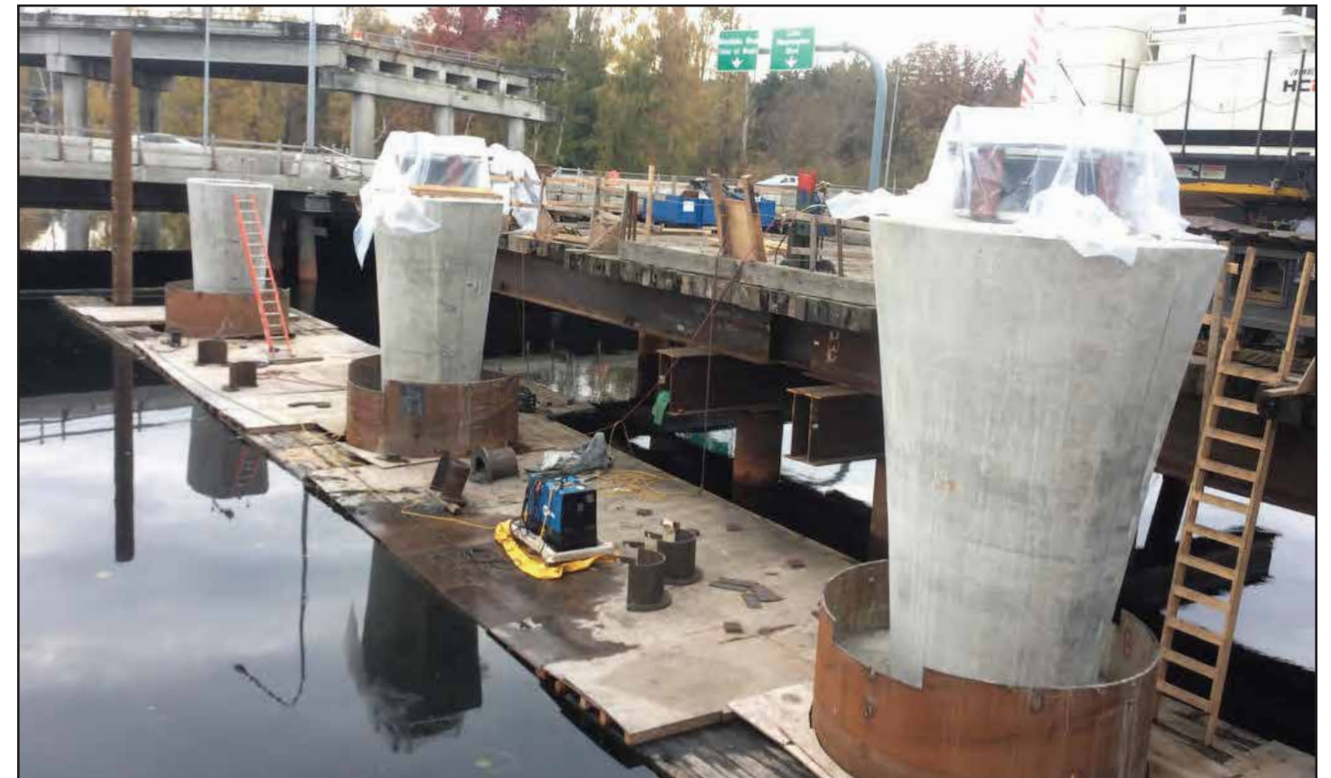
Concrete columns for the West Approach Bridge North are topped with seismic isolation bearings, which allow each section of the bridge to move independently during an earthquake. Photo taken: Nov. 17
