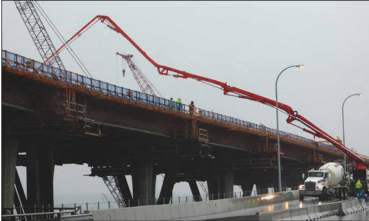
During a Dec. 9-12 closure of SR 520, crews pour concrete for eastern spans of the West Approach Bridge North, near the new floating bridge. Photo taken: Dec. 10
