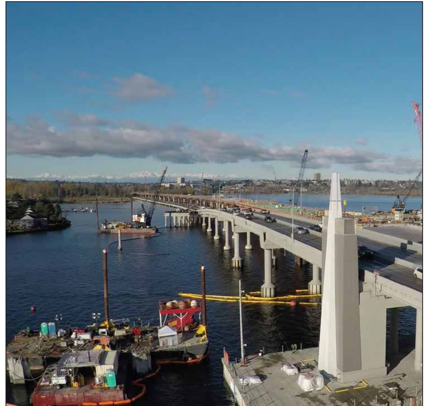
Decommissioning of the old floating bridge nears completion as crews (lower left) remove the final underwater piece of concrete column that supported a segment of the old west approach bridge. Photo taken: Dec. 8
