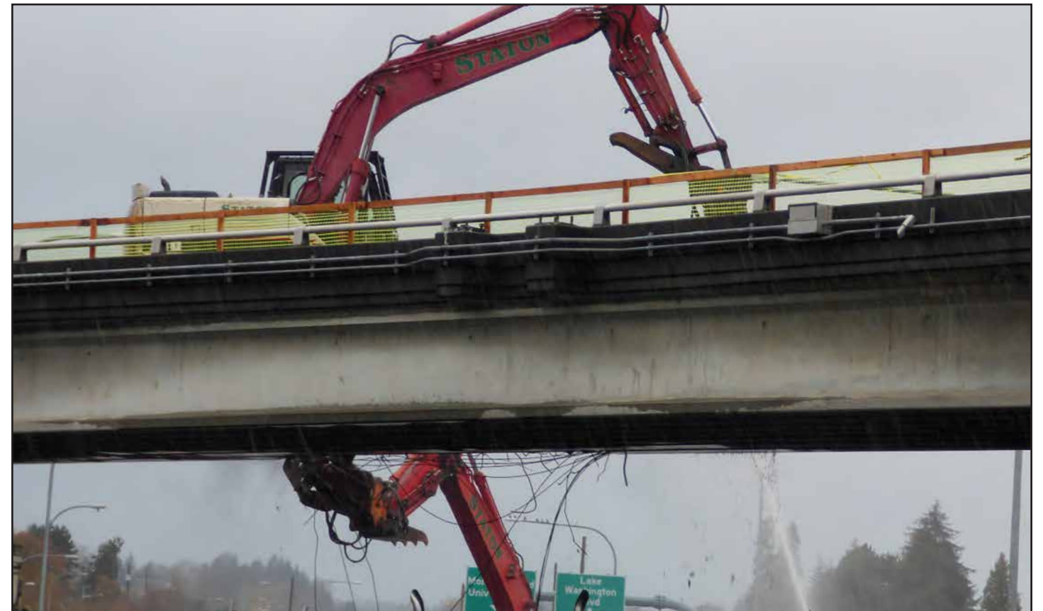
During a Dec. 9-12 closure of SR 520, excavator operators remove part of the old westbound SR 520 off-ramp to Lake Washington Boulevard. The old ramp crossed over the SR 520 mainline. Photo taken: Dec. 10
