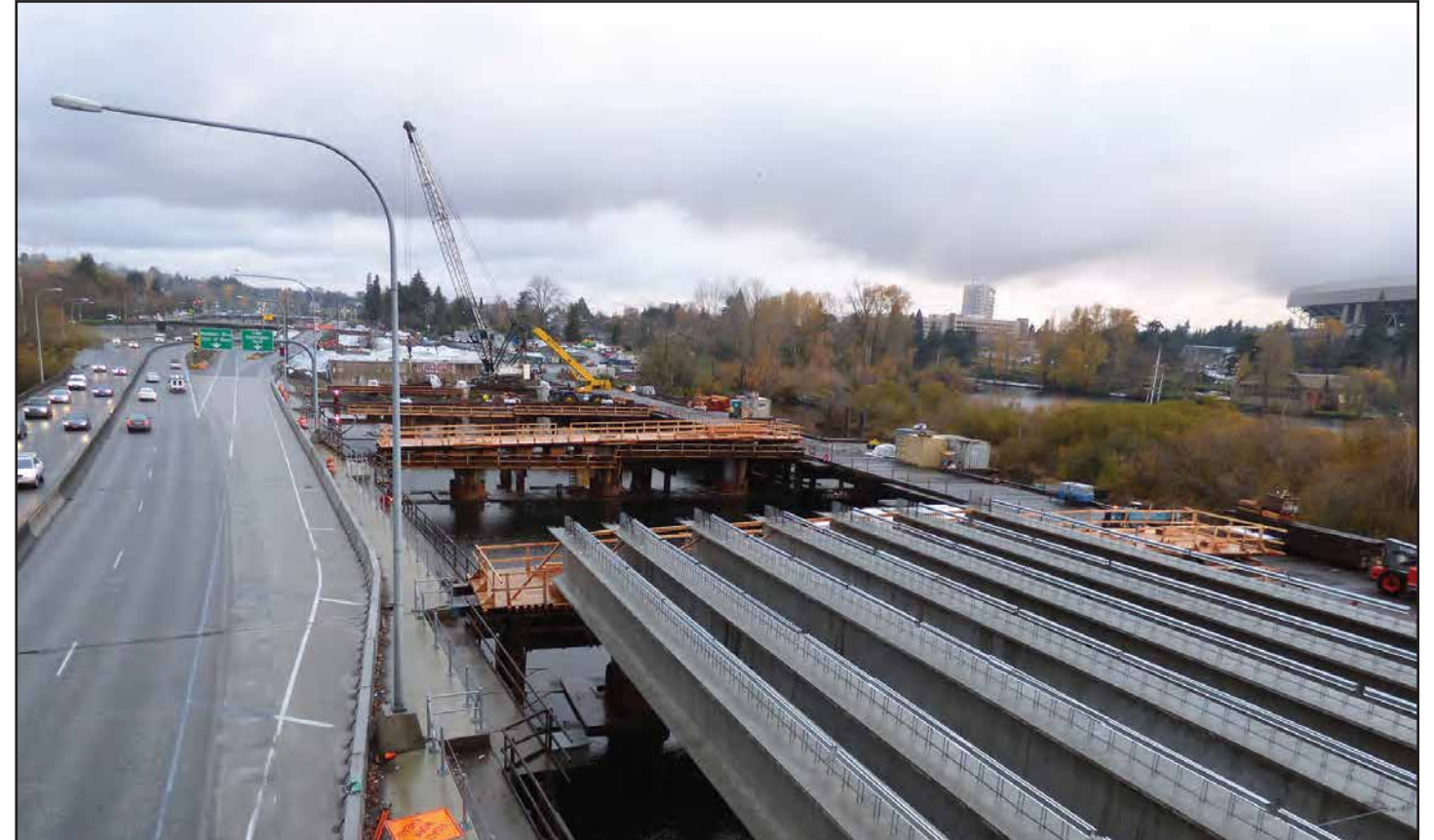
After months of nighttime girder deliveries and installations, crews close in on completing girder placements in Montlake at the west end of the new, 1.2-mile-long West Approach Bridge North. Photo taken: Dec. 5
