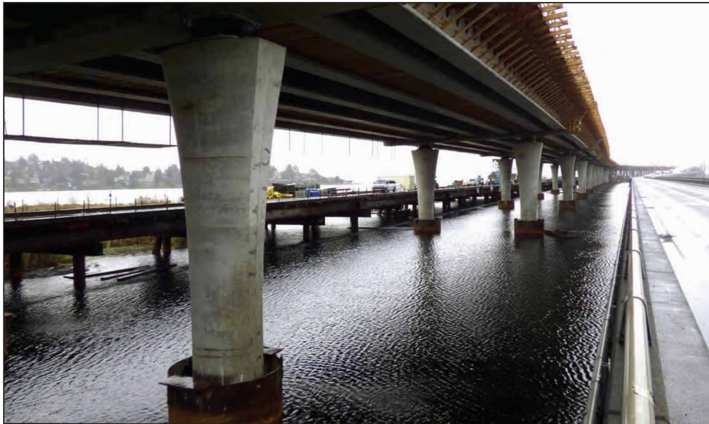
Fluted concrete columns for the new West Approach Bridge North stretch eastward toward the new floating bridge. Photo taken: Dec. 10
