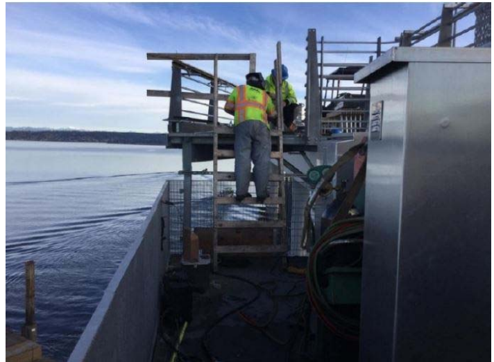
WABN: Shared-use path gate panels at Pier 28 belvedere
