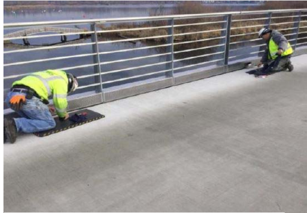
WABN: Labeling lights on the shared-use path
