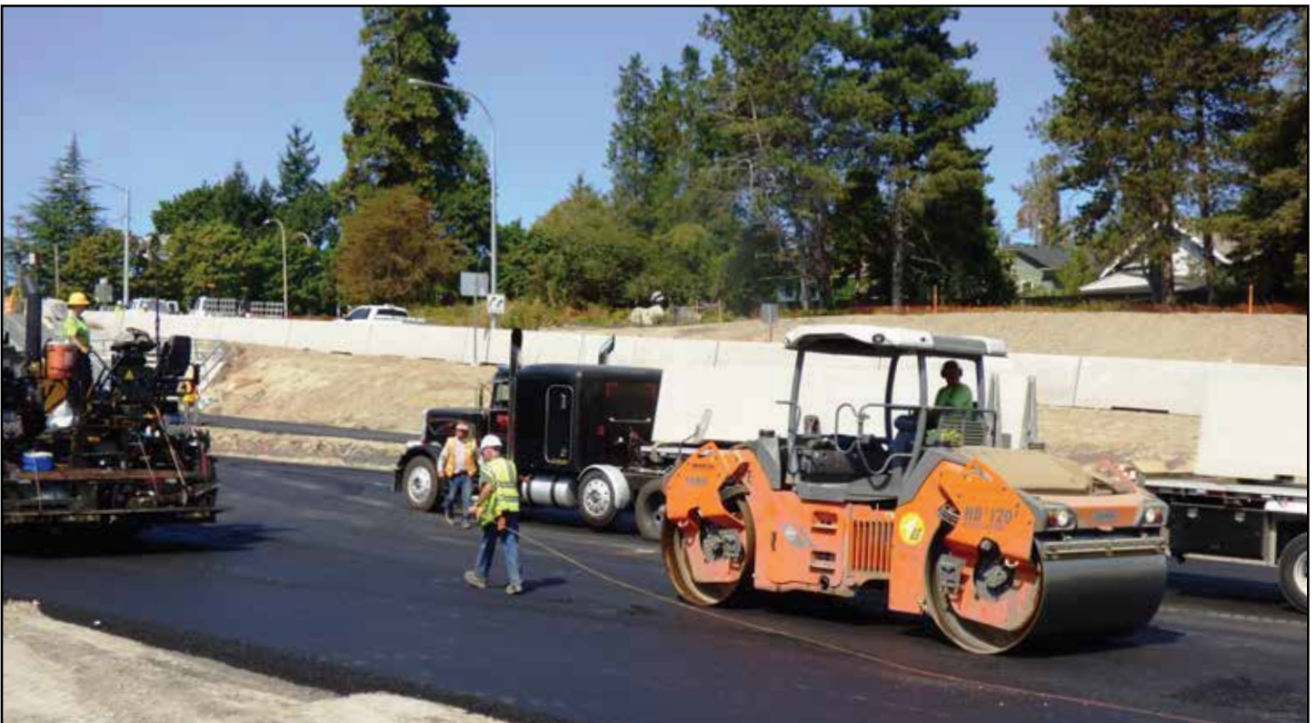
A worker marks the new westbound SR 520 lanes in preparation for roadway striping during the August 2017 weekend closure of SR 520.
