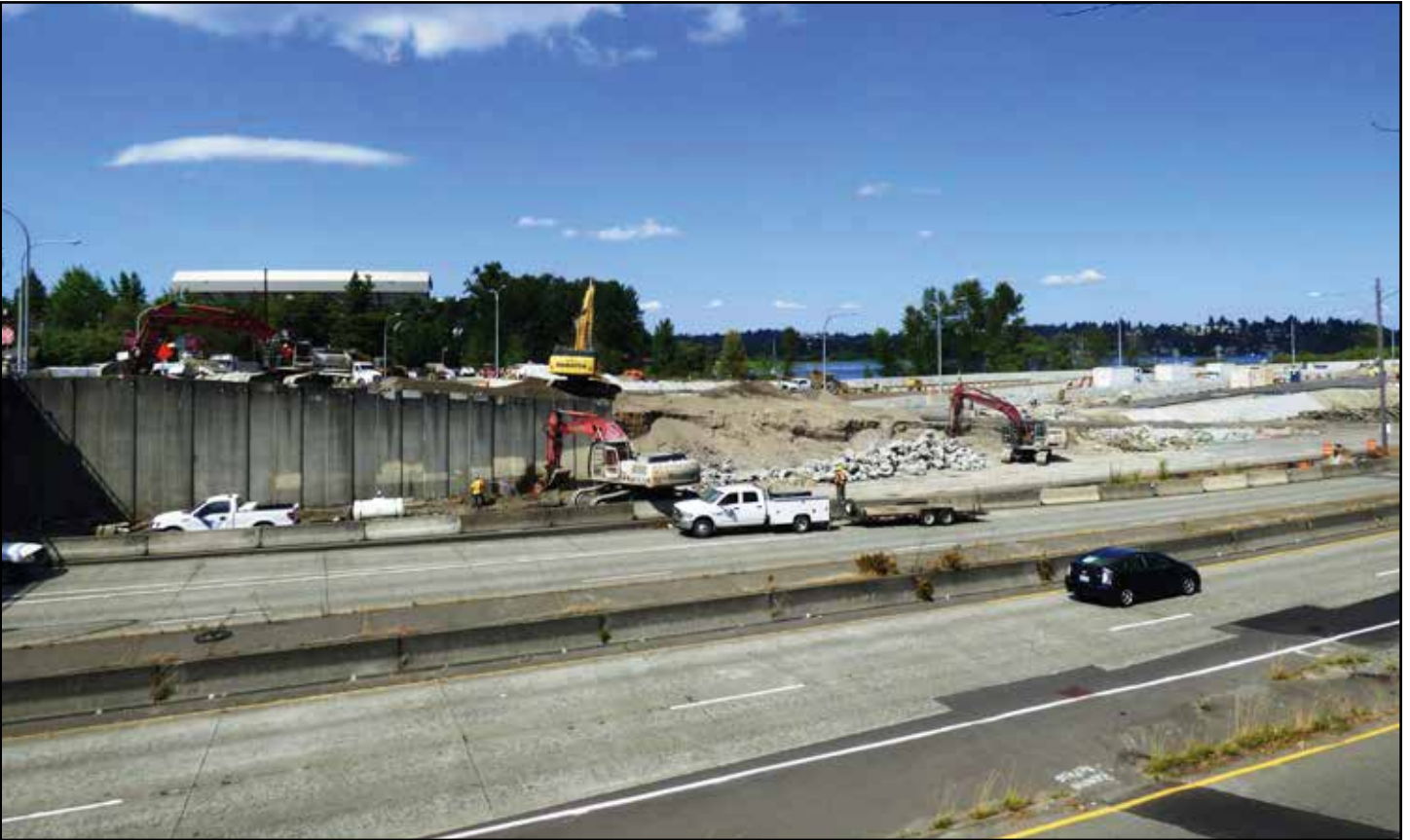
During the July 2017 weekend closure of SR 520, crews remove a retaining wall that separated the old westbound SR 520 lanes from the former location of the Museum of History and Industry.
