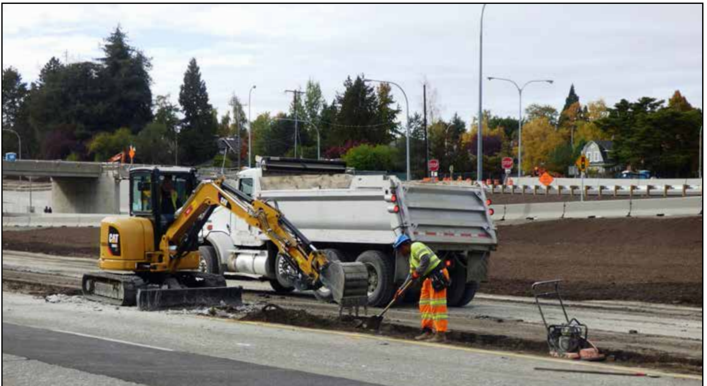
Workers remove material from an old drainage ditch to prepare it for paving during an October 2017 closure of eastbound SR 520.
