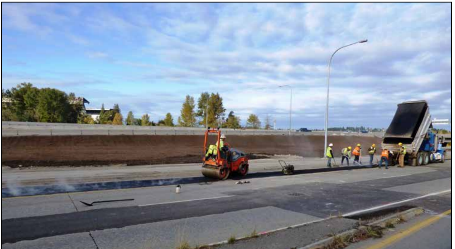
During an eastbound SR 520 closure in October 2017, crews repaved sections of the roadway. Here, crews place and spread asphalt, and compact and smooth the fresh asphalt to repair a drainage ditch.
