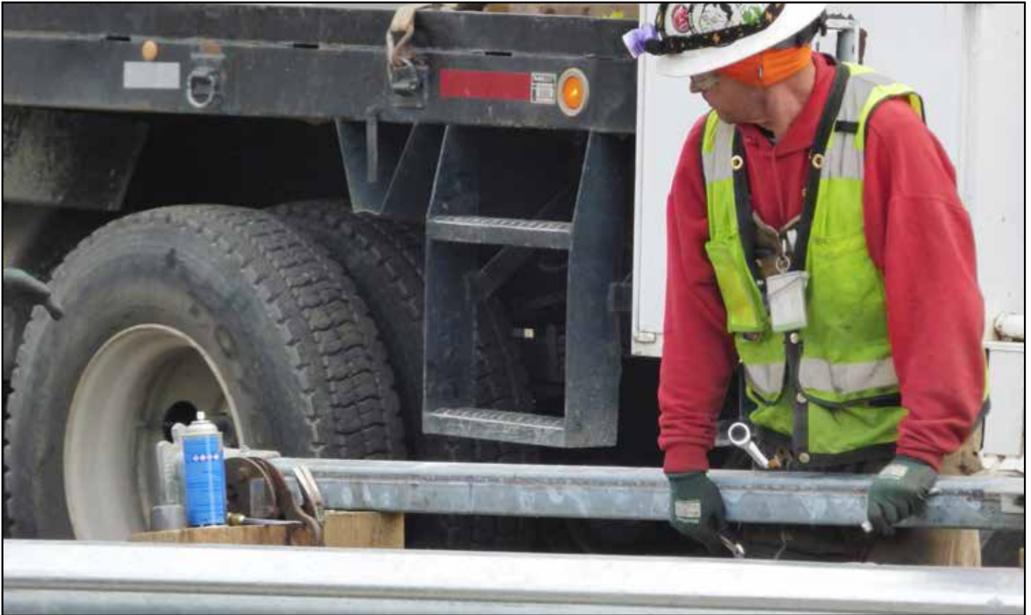
During a weekend closure of eastbound SR 520 in October 2017, a crewmember works on the mounting bolts for a sign post.
