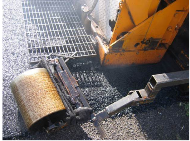
Figure 19. Close-up of roller hardware.
