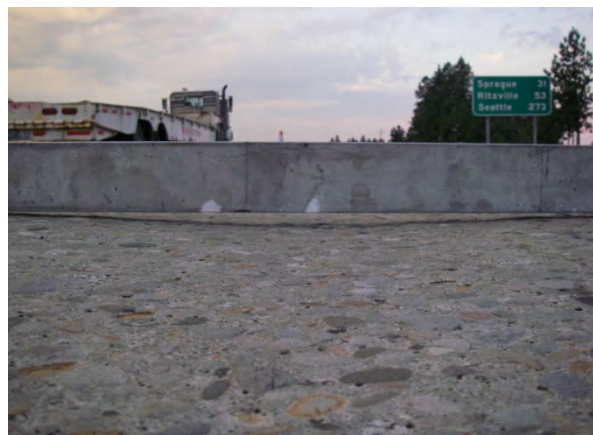
Figure 30. Amount of wear in rut fill section.
