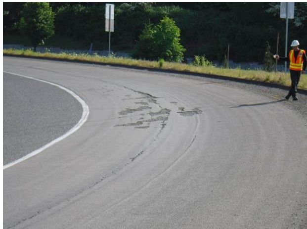
Figure 36. Delamination across lane.
