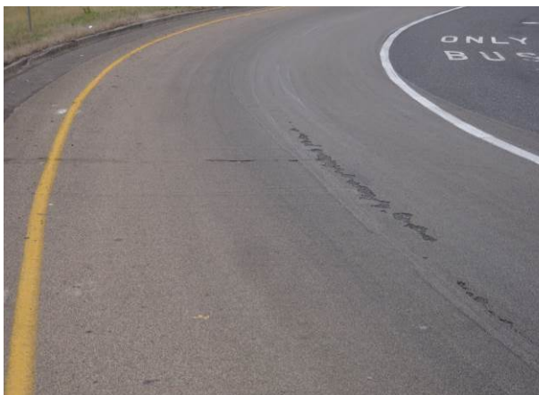
Figure 31. Wheel path delamination.
