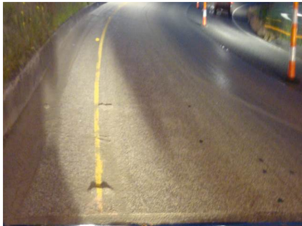
Figure 25. Excess aggregate on overlay.
