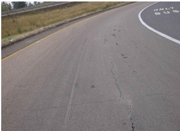
Figure 29. Longitudinal and transverse cracking and minor delamination.
