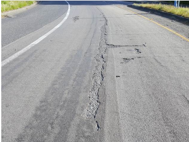
Figure 33. Wheel path delamination.
