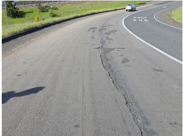
Figure 34. Wheel path delamination.
