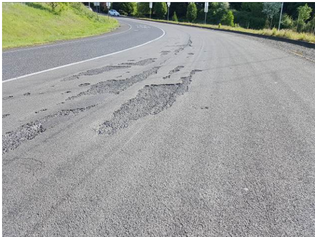
Figure 35. Delamination across lane.
