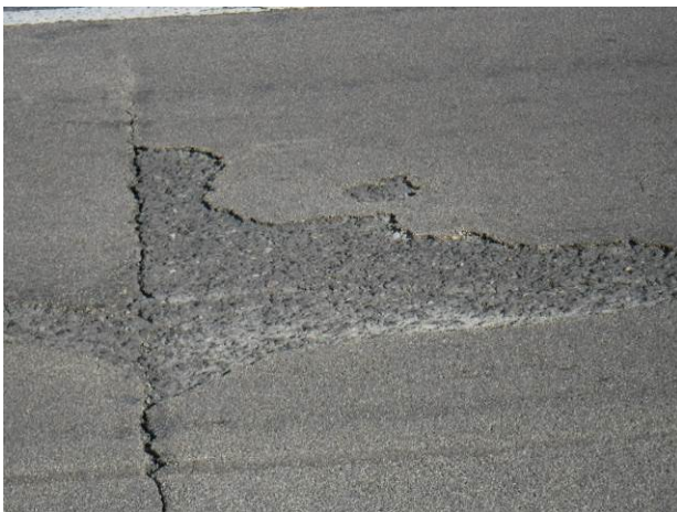
Figure 37. Delamination and transverse crack.
