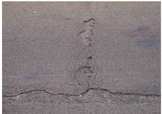
Figure 30. Transverse crack and delamination.
