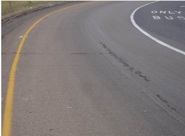
Figure 27. Longitudinal joint delamination.
