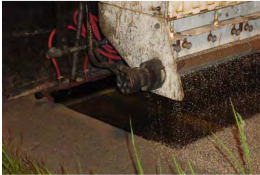
Figure 20. Close-up of spreader bar distributing epoxy binder and aggregate spreader dropping material on top of the epoxy.
