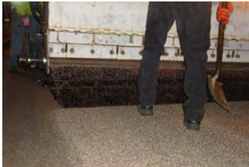
Figure 19. Aggregate being applied to epoxy after being placed on the pavement surface.
