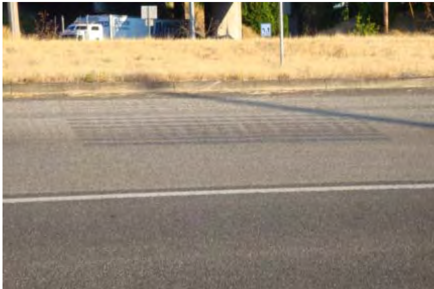
Figure 13. Streaking in aggregate coverage.
