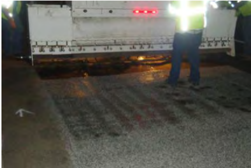
Figure 10. Streaking surface caused by inconsistency of the aggregate spreader.
