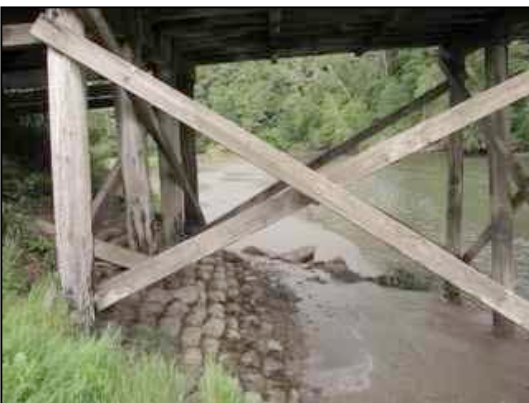
Figure 22. Bank under structure on north side
