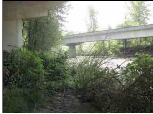
Figure 115. Thick vegetation through median
