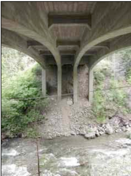
Figure 59. Steep bank on west side
