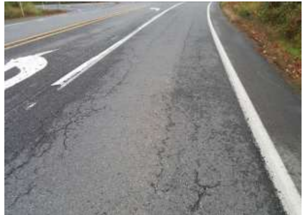
Figure 41. Open-texture, raveling, alligator and longitudinal cracking at MP 14.6. (93117)
