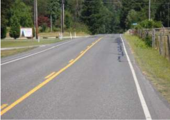
Figure 31. Sealed alligator cracking at MP 17.24. (6593)
