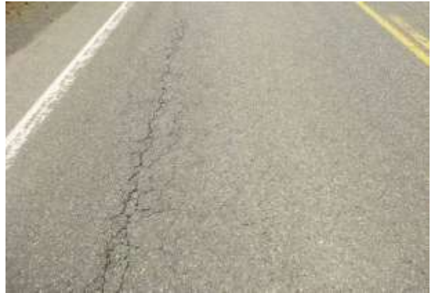
Figure 22. Pre-construction alligator cracking. (1363)
