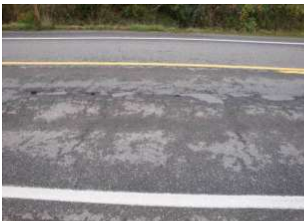
Figure 46. Alligator and transverse cracking and potholes at MP 17.3. (00562)
