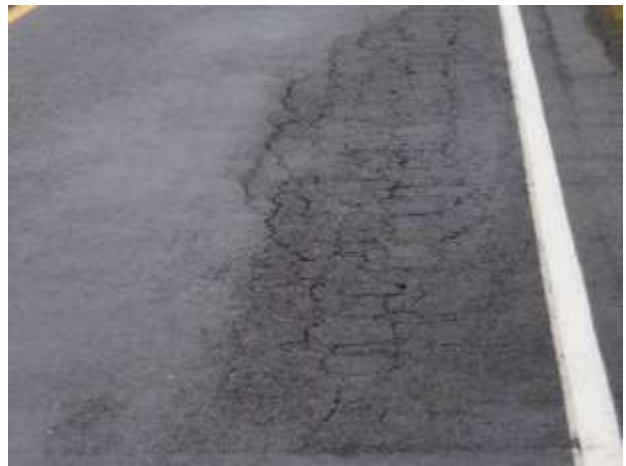
Figure 30. Close-up of alligator cracking at MP 17.2. (4870)
