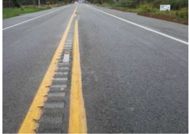
Figure 37. Open-texture and raveling at MP 10.1. (90232)
