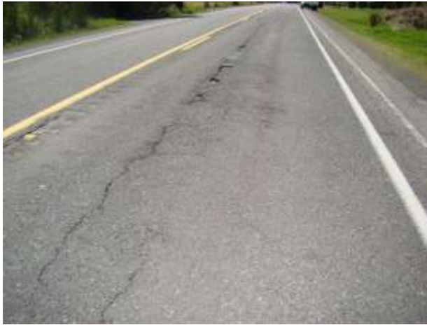
Figure 34. Alligator, longitudinal cracking and potholes in the westbound lane at MP 17.2 in May 2013. (1334)
