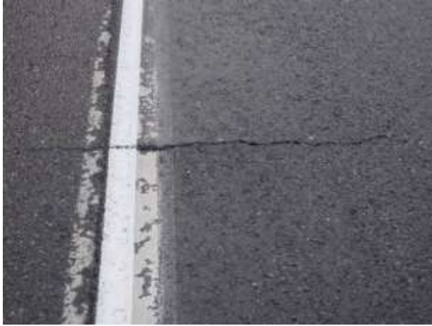
Figure 27. Transverse crack at MP 14.10. (4826)
