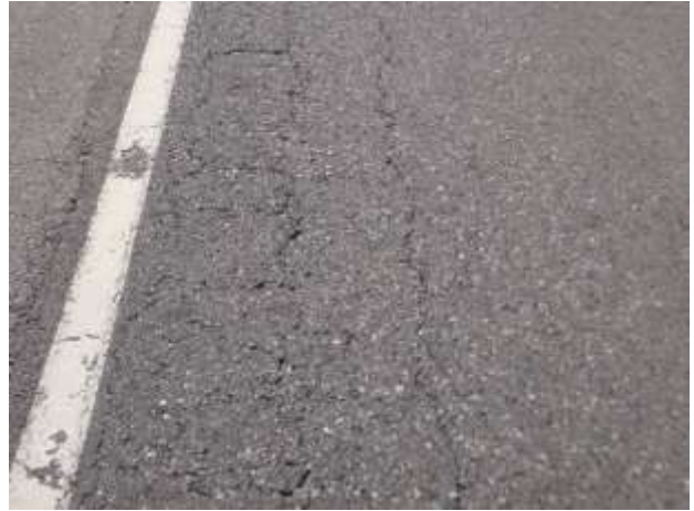
Figure 32. Alligator and long. cracking at unknown location. (6594)
