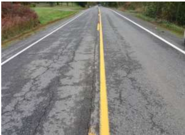
Figure 44. Alligator and longitudinal cracking at MP 17.3. (94210)
