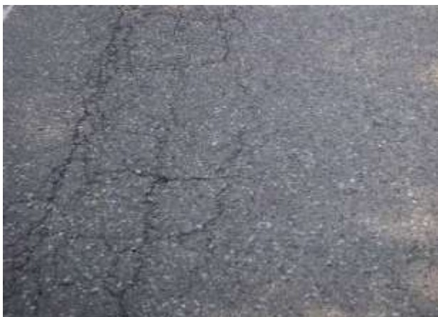
Figure 25. Pre-construction alligator and longitudinal cracking. (1366)
