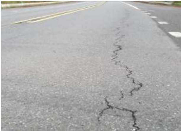
Figure 40. Open-texture, raveling, alligator and longitudinal cracking at MP 14.1. (92525)
