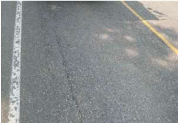
Figure 21. Pre-construction longitudinal cracking. (0776)
