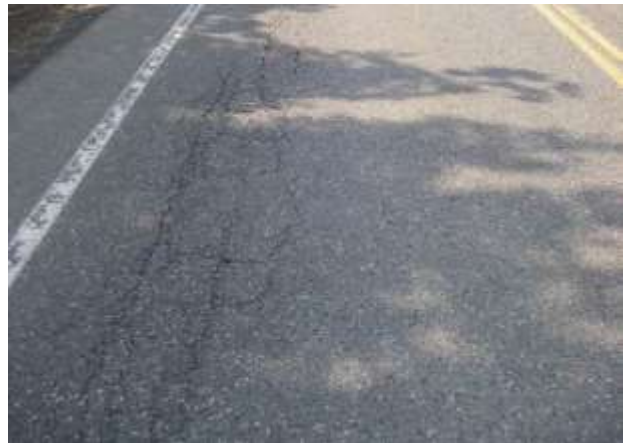
Figure 24. Pre-construction alligator and longitudinal cracking. (1365)
