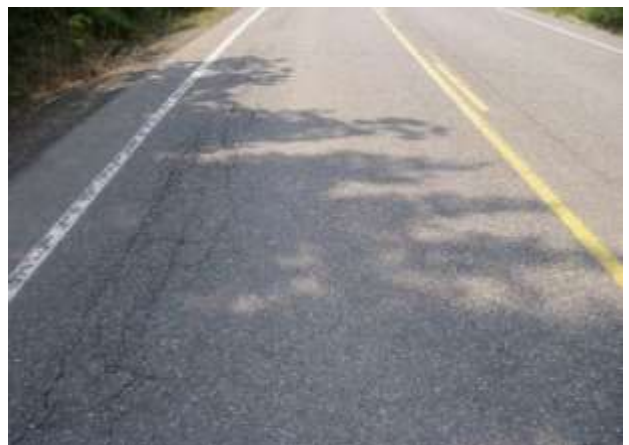
Figure 26. Pre-construction alligator and longitudinal cracking. (1367)
