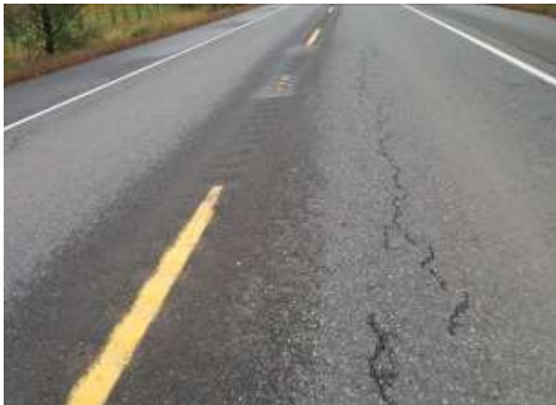
Figure 38. Open-texture, raveling and longitudinal cracking at MP 11.8. (90910)
