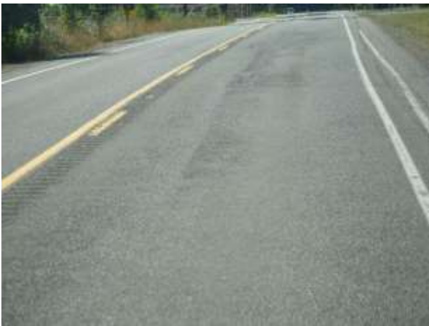
Figure 33. Alligator cracking at unknown location. (6590)
