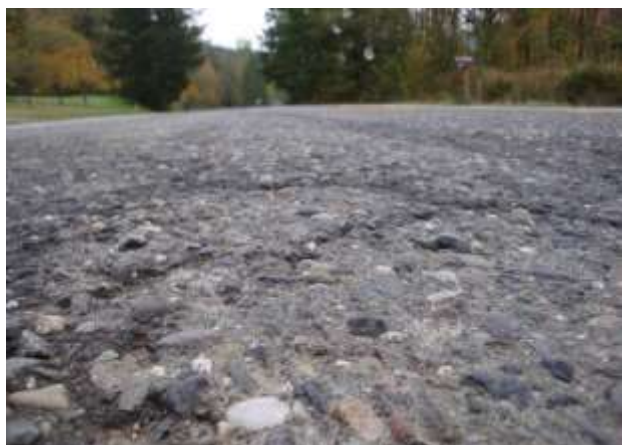
Figure 47. Close-up of raveled surface of pavement at MP 17.3. (00559)
