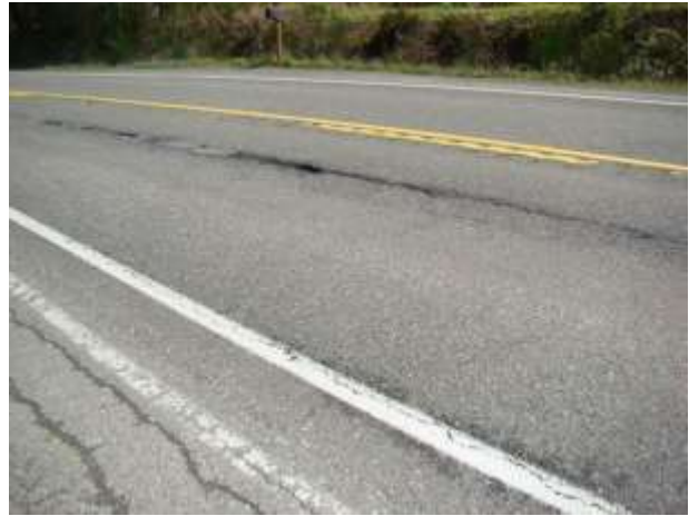
Figure 35. Alligator, longitudinal cracking and potholes in the westbound lane at MP 17.2 in May 2013. (1335)
