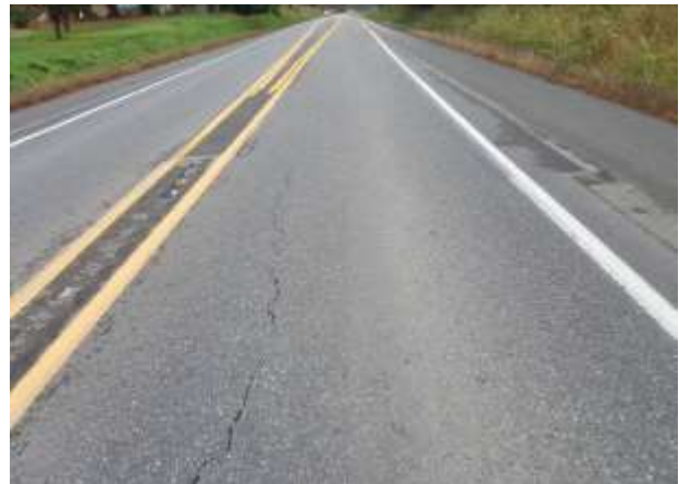
Figure 39. Open-texture, raveling and longitudinal cracking at MP 13.15 (90910)
