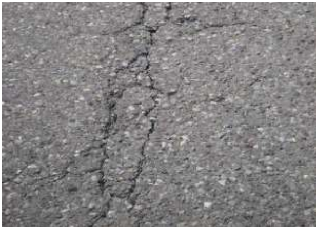
Figure 23. Pre-construction alligator cracking. (1364)
