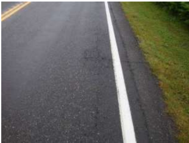
Figure 29. Alligator and longitudinal cracking at MP 17.2. (4807)
