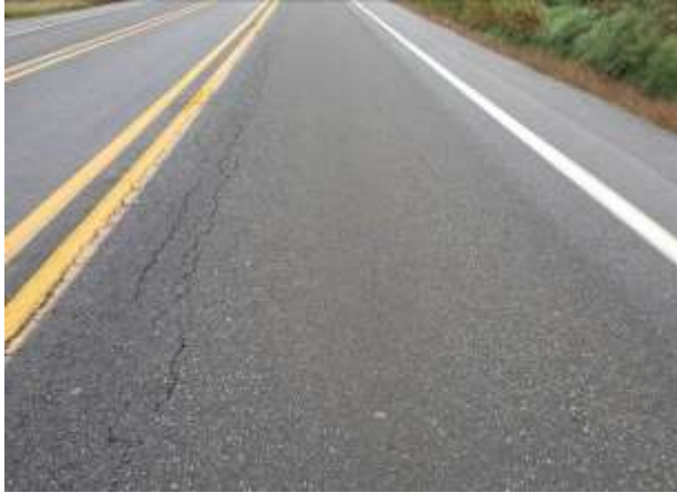
Figure 36. Longitudinal and alligator cracking at MP 4.8. (85258)
