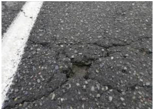
Figure 45. Alligator cracking, raveling and pothole at MP 17.3. Note erosion of the binder surrounding the aggregate. (94527)
