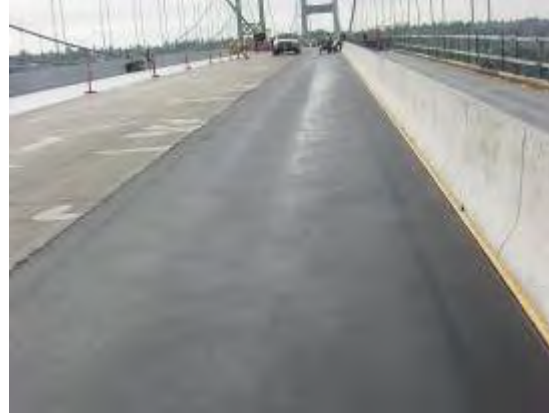
Figure 36. Flushing in Lane 1 several days after paving.
