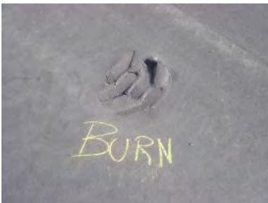
Figure 37. Indentation in base course left by equipment tire.
