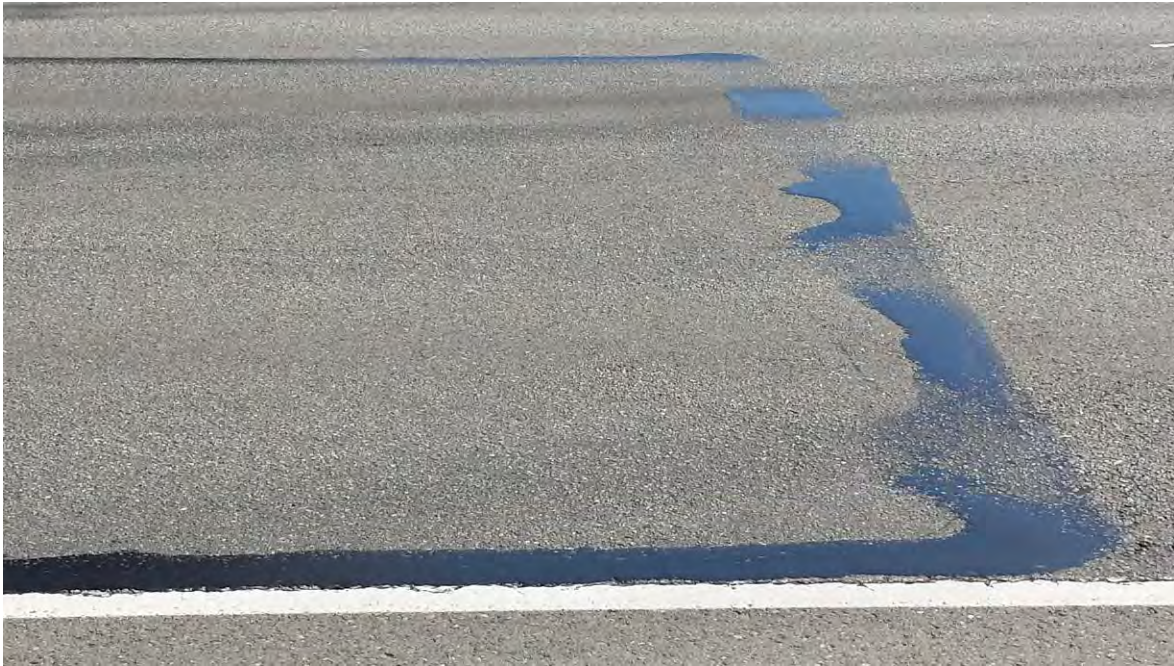
Figure 62. Close-up of HMA patch showing minimal raveling in the wheel paths. (Photos from 5/1/14)
