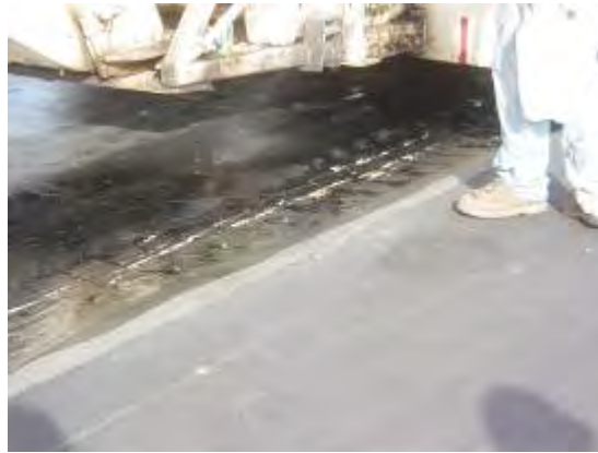
Figure 21. Adhesion layer damaged by track.
