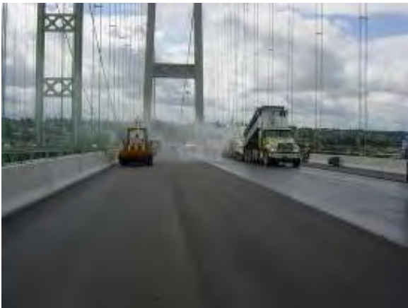
Figure 33. Streaks in top course on Lanes 4 and 5.
