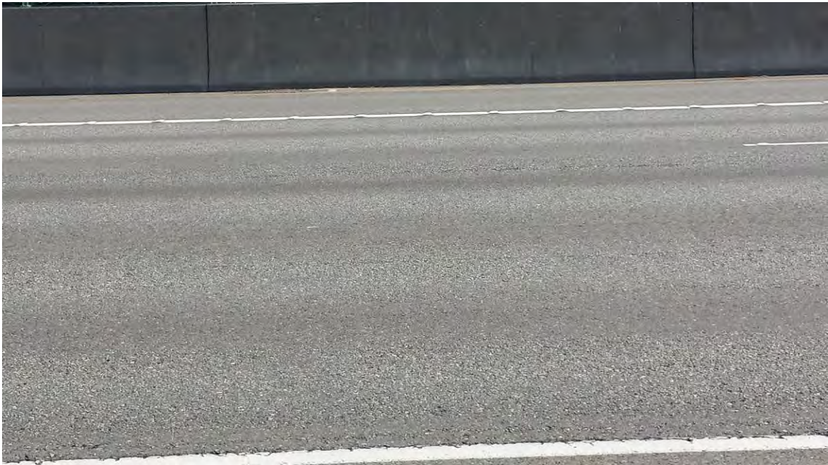
Figure 56. Moderate raveling in all lanes. (Photo from 5/1/2014)
