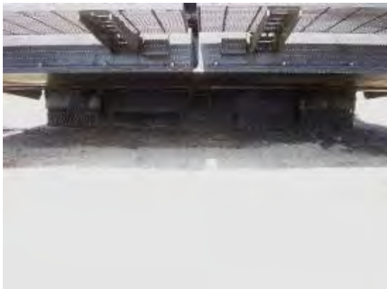
Figure 13. Missing chains on MMK retrofit on I-R/Blaw-Knox PF-4410 paver.
