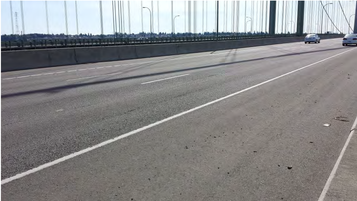
Figure 54. Severe raveling in the wheel paths of Lane 1. Note linear nature of the raveling in left wheel path of Lane 1. (Photo from 5/1/2014)
