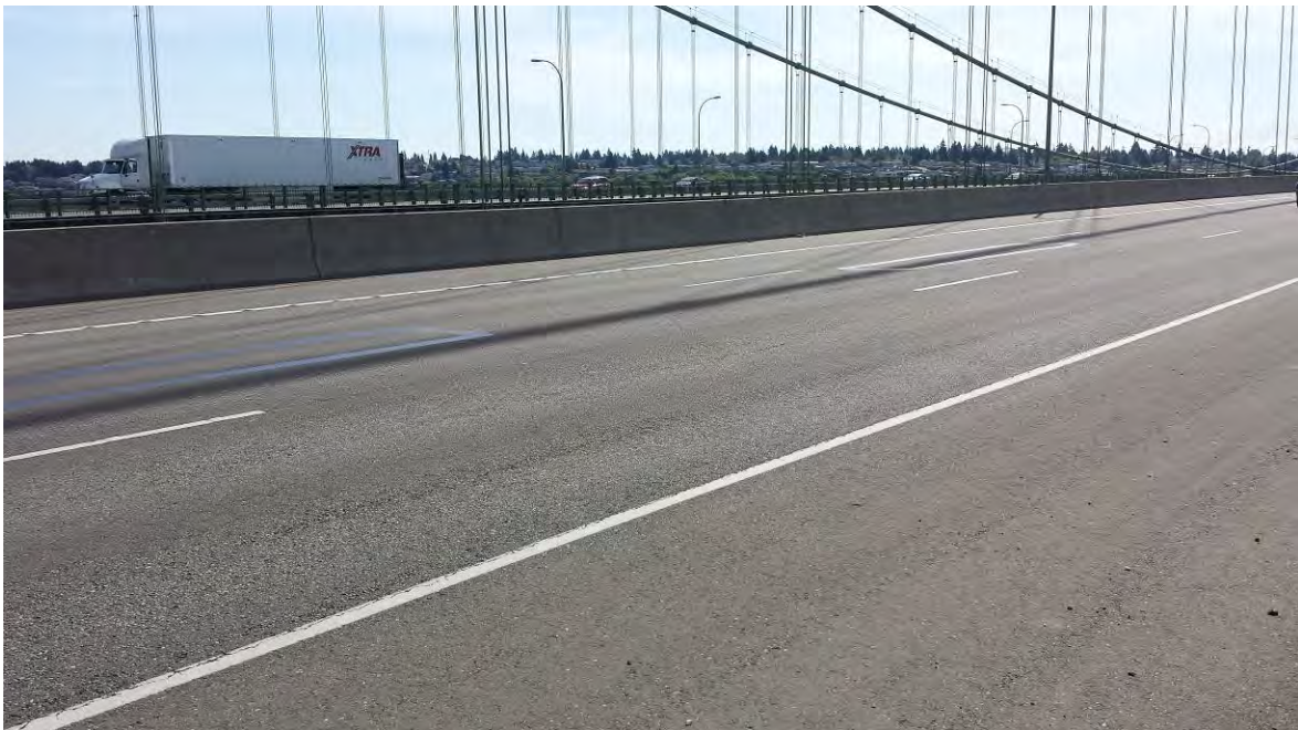
Figure 55. Severe raveling in Lane 1, patch in Lane 2. (Photo from 5/1/2014)
