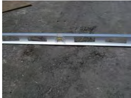
Figure 42. Possible repaired area.
