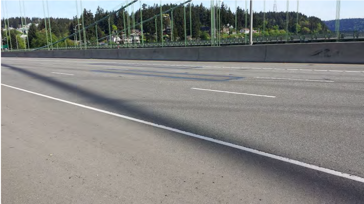
Figure 58. Patches in Lanes 2 and 3. (Photos from 5/1/14)
