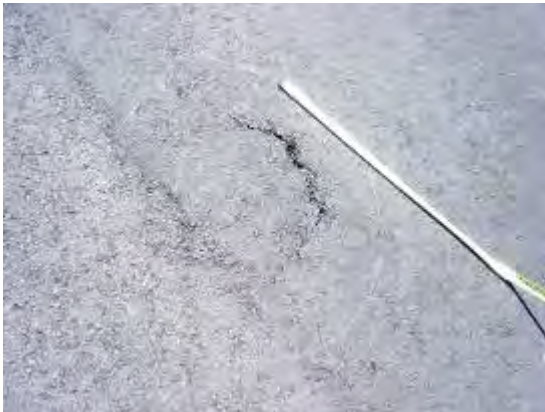
Figure 41. Indentation with crack near midspan.
