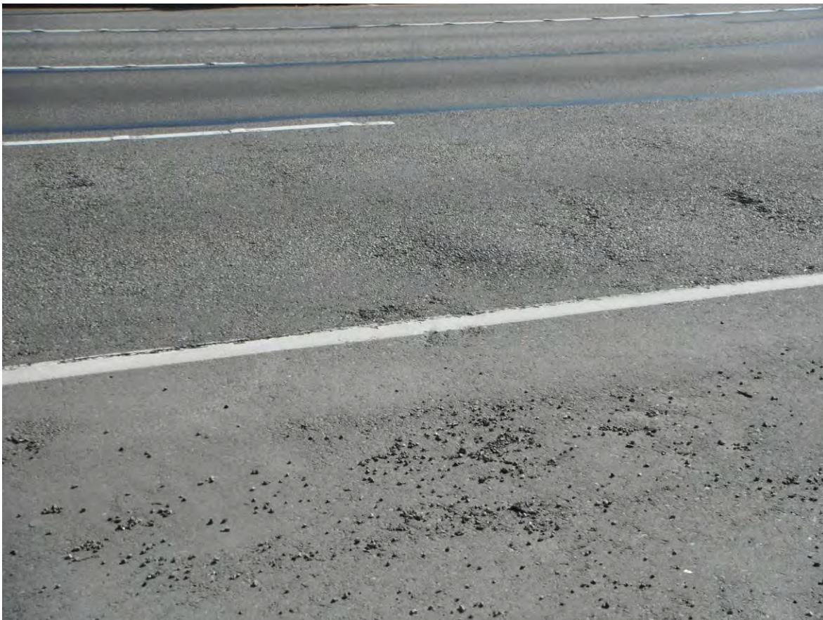
Figure 53. Severe raveling in the wheel paths of Lane1 and patch in Lane 2. Note accumulation of gravel on the shoulder. (Photo from 5/1/2014)
