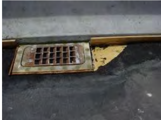
Figure 23. Triangle of adhesion layer removed near scupper due to water damage.
