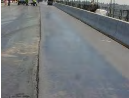
Figure 35. Flushing in Lane 1 immediately after paving.
