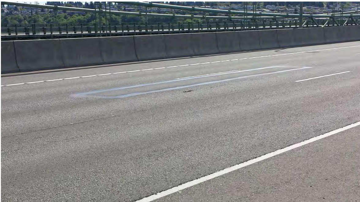
Figure 59. Patch and severe raveling in Lane 2. (Photos from 5/1/14)
