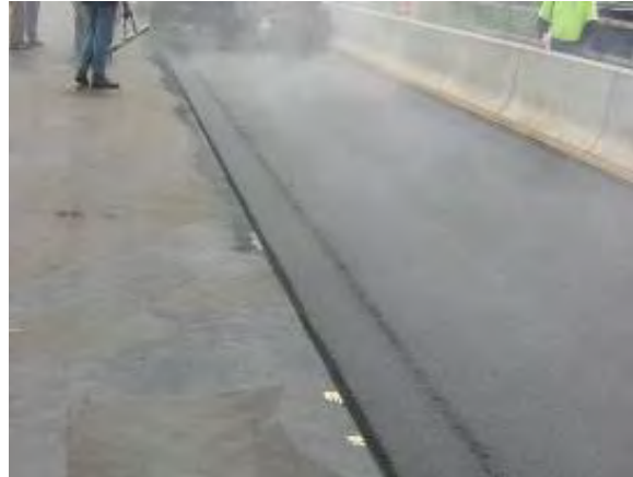
Figure 34. Streak left by screed extension.
