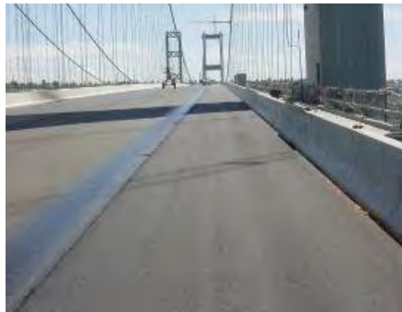
Figure 32. Streaks in top course on Lane 1.
