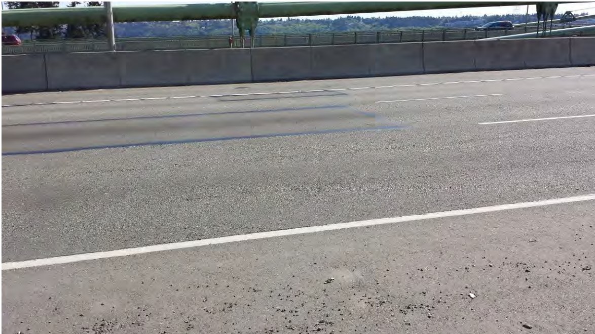
Figure 60. Severe raveling Lane 1, patches Lanes 2 and 3. (Photos from 5/1/14)
