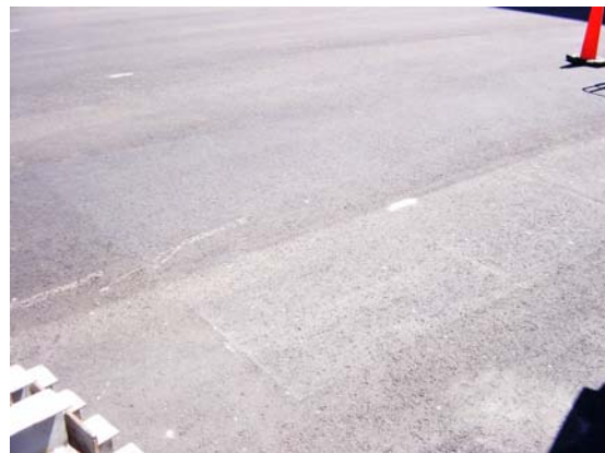
Figure 40. Indentation left by Demag crane pad.
