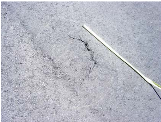
Figure 41. Indentation with crack near midspan.
