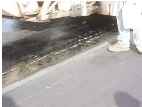
Figure 21. Adhesion layer damaged by track.
