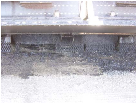
Figure 12. Missing chains on MMK retrofit.
