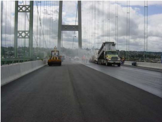
Figure 33. Streaks in top course on lanes four and five.
