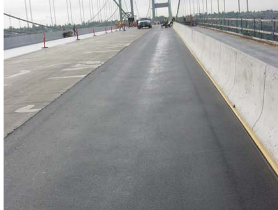
Figure 36. Flushing in lane one several days after paving.
