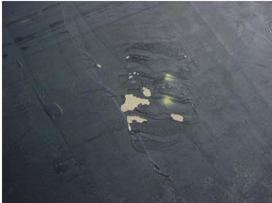
Figure 7. Damage to adhesion layer.
