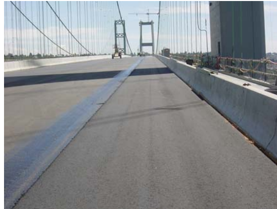
Figure 32. Streaks in top course on lane one.
