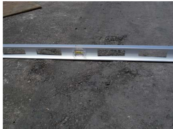
Figure 42. Possible repaired area.
