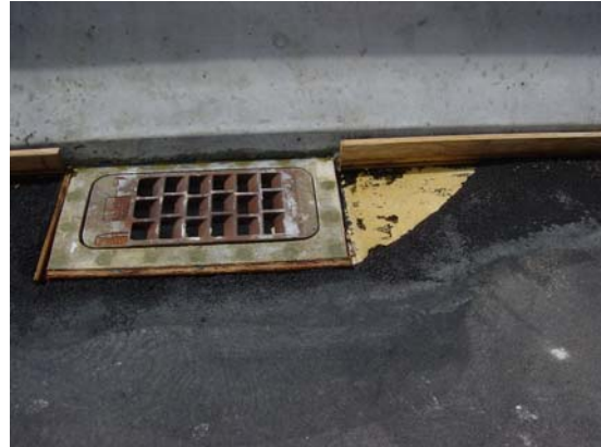
Figure 23. Area removed near scupper due to water damage.
