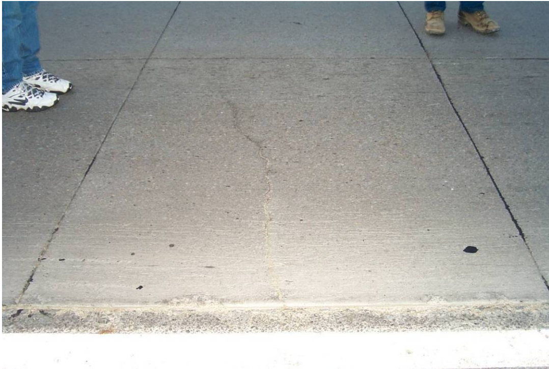
Figure 16. Mid-panel transverse crack in 5 inch test section.
