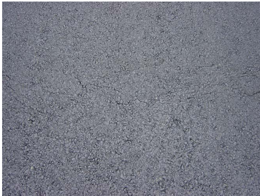
Figure 4.7: Cracking problems in test section number 8.
