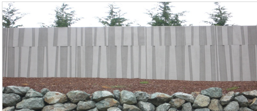
Context-appropriate walls used to blend the adjacent forested character with the Built environment where there is no longer room for vegetation. Simple, large-scale patterns are effective at freeway speeds.
