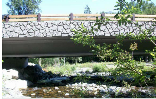
Texturing on the outside of bridges can be used when there are anticipated viewers from this perspective.
