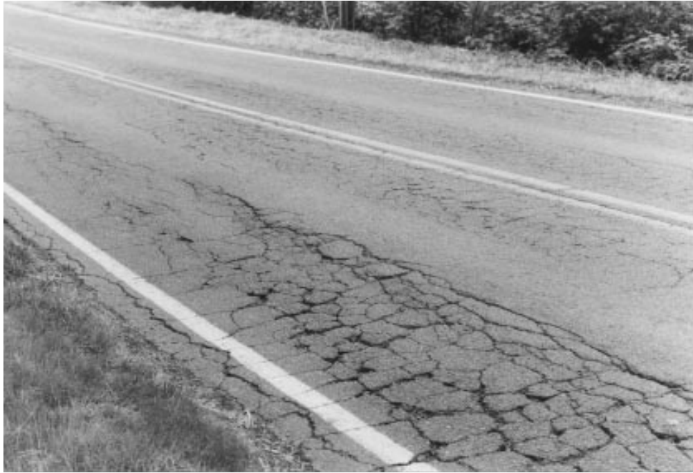
Alligator cracking is a common pavement distress noted during a pavement condition evaluation.
