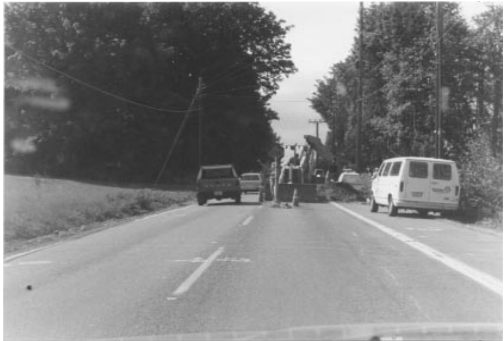
A backhoe is used for a test pit to get information about the material underlying the roadway.
