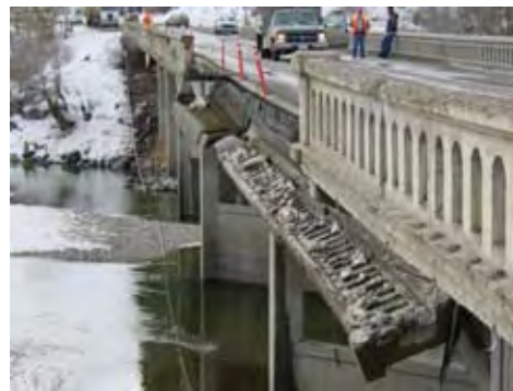
BEFORE: Nonstandard bridge rail on SR153 near Carlton, Washington. This illustrates the safety risk posed by nonstandard bridge rail
