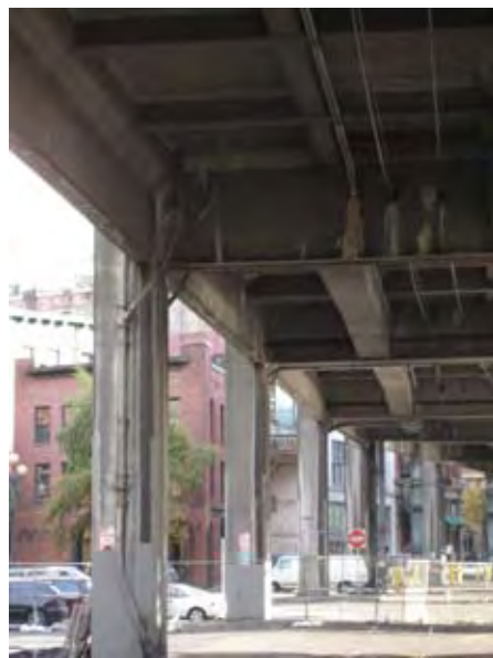
Crews began work to stabilize four viaduct column footings on the Alaskan Way Viaduct between Columbia Street and Yesler Way
