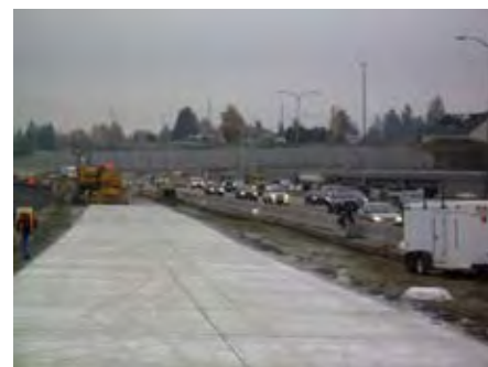
A new four-lane collector-distributor opened on northbound I-5 in Tacoma on December 8
