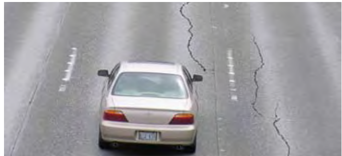
Cracked and rutting PCC pavement on I-5 through Seattle at NE 130th St.
