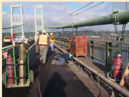
Crews remove the existing rub rail on the north side of the 1950 bridge.
