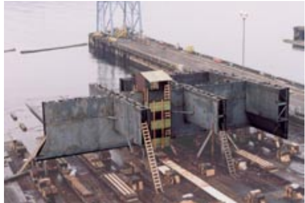
Approximately one quarter of the first caisson “cutting shoe” is shown complete in this recent photo. It will be placed at the base of the tower indicated above.
