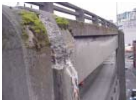
Damage at Bent 100
