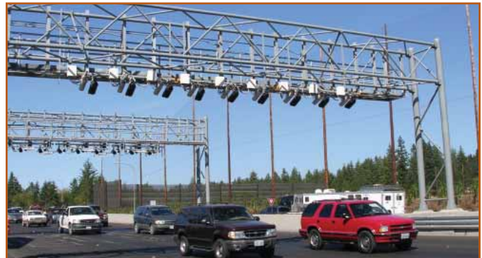
Tolling gantries, located over the highway, read transponders and license plates, without causing drivers to slow down.
