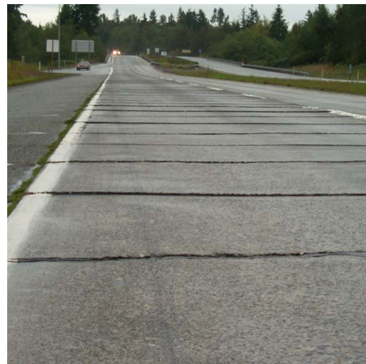
Faulted concrete pavement.
