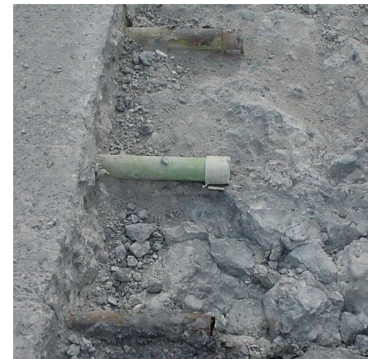
Corroded epoxy coated dowel bars.
