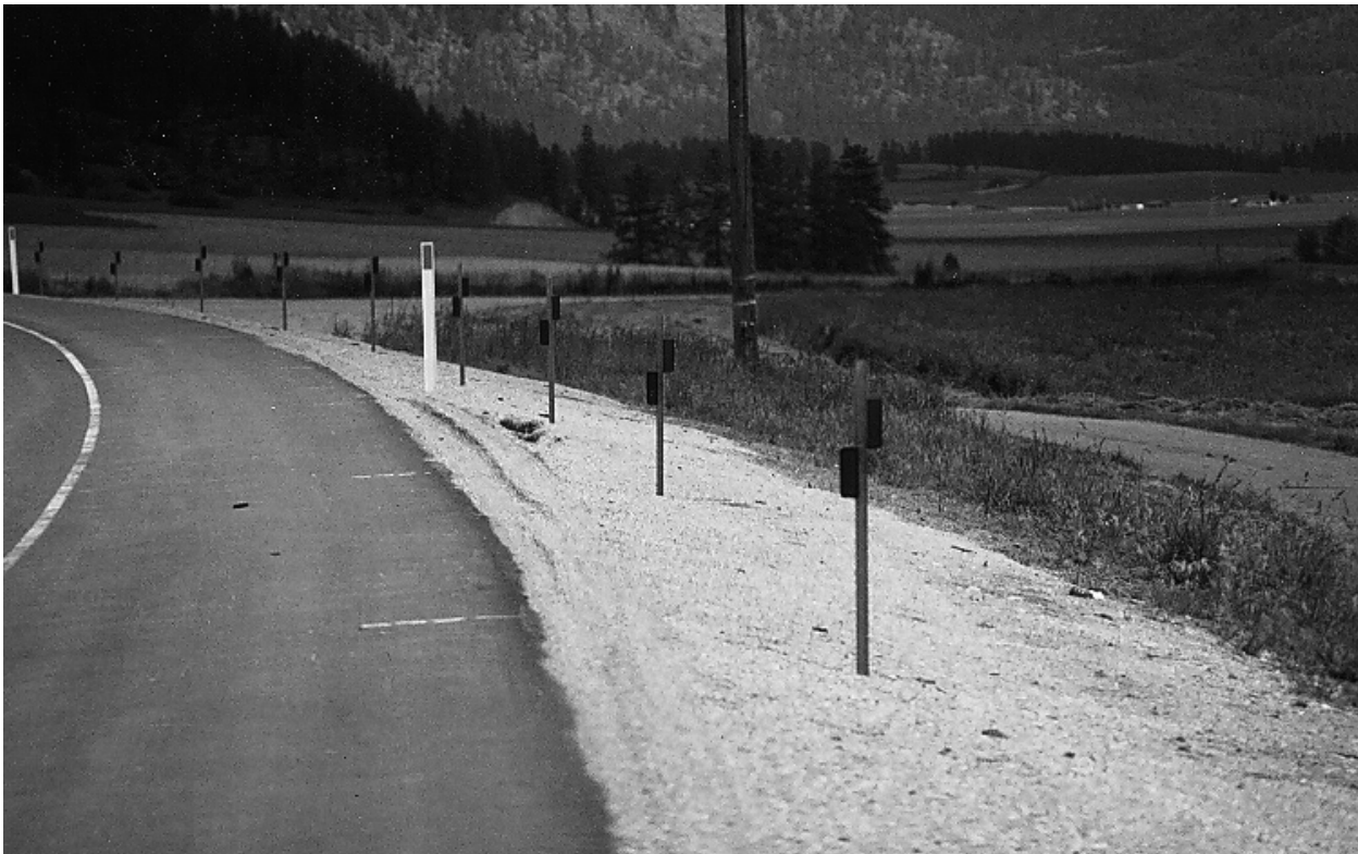
Wildlife Reflectors on the Outside of a Curve Figure 830-4
