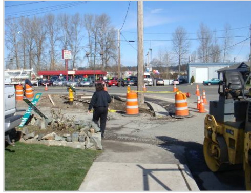
Does not meet ADA requirements
