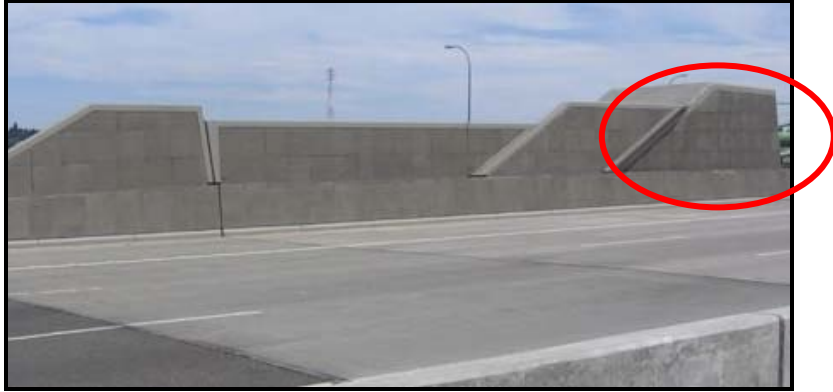
New walls with absorptive treatment, walls on NW corner of bridge. Cable housing circled in red for comparison with images below.
