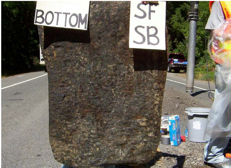
Figure 3.26. Bottom of SF-SB geotextile after removal.
