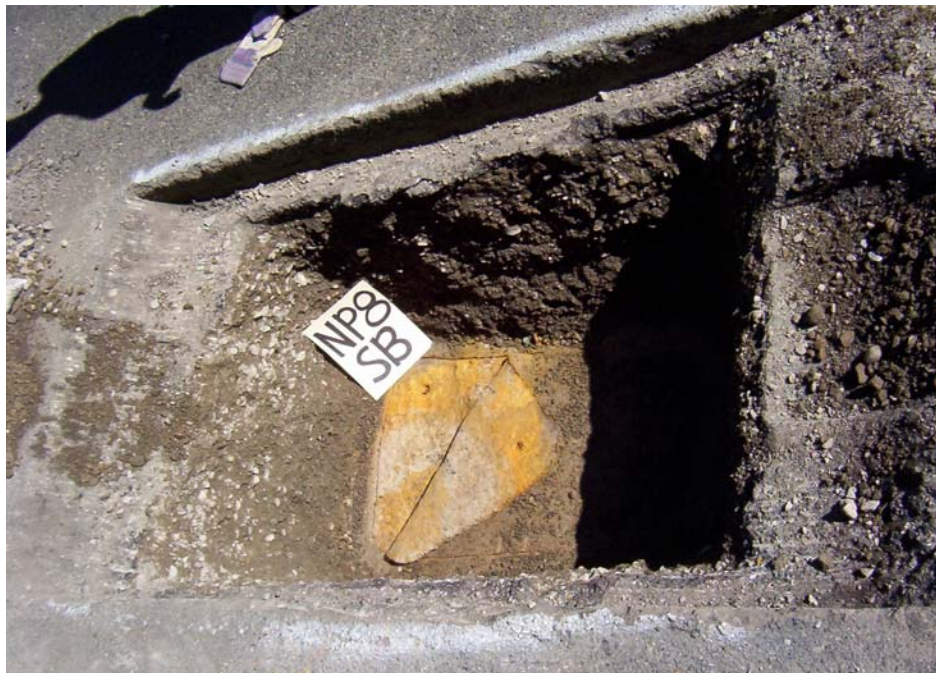
Figure 3.22. NP8-SB test pit with geotextile peeled back.
